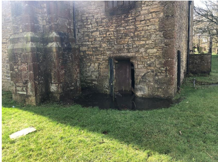
P11 (4627): Flooded basement/ damaged door
