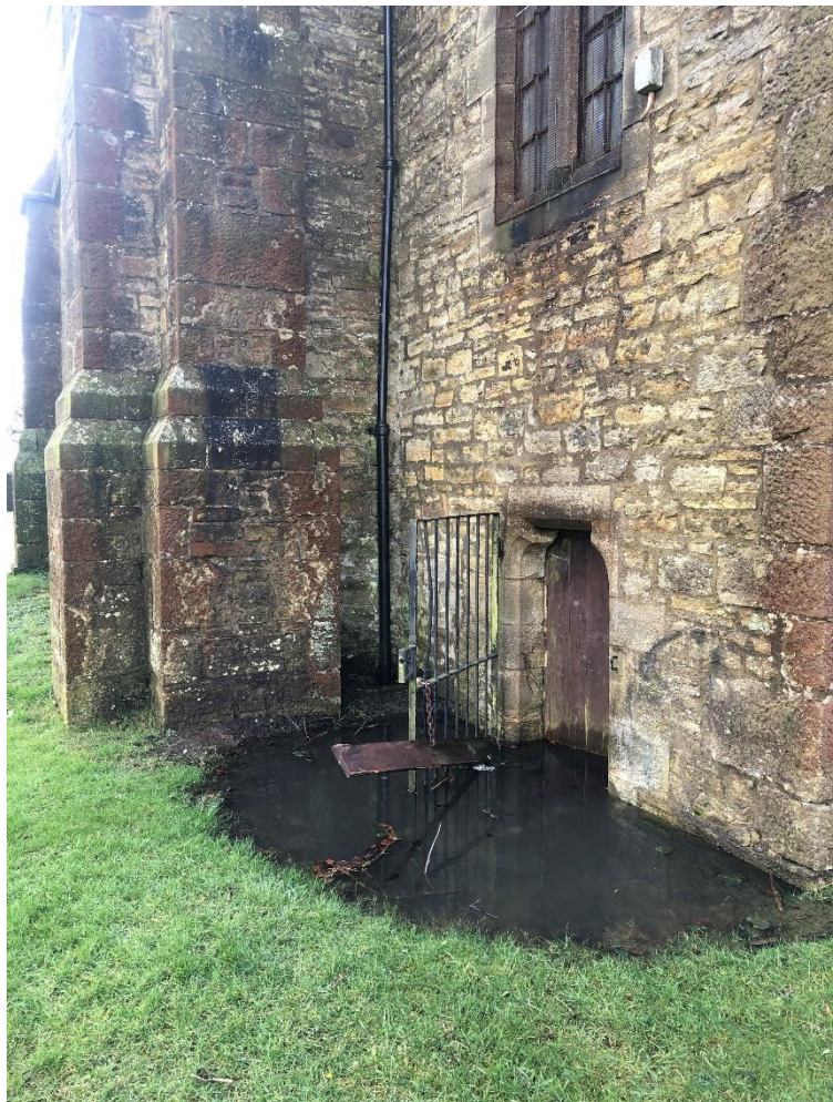
P12 (4628): Flooded basement/ damaged door (side view)
