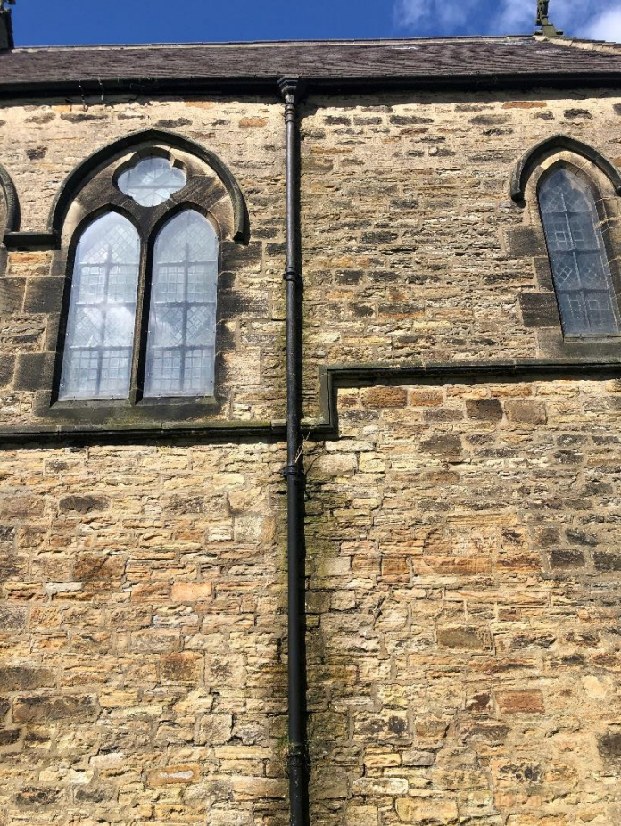
P7 (4793): Chancel south wall, water seepage
