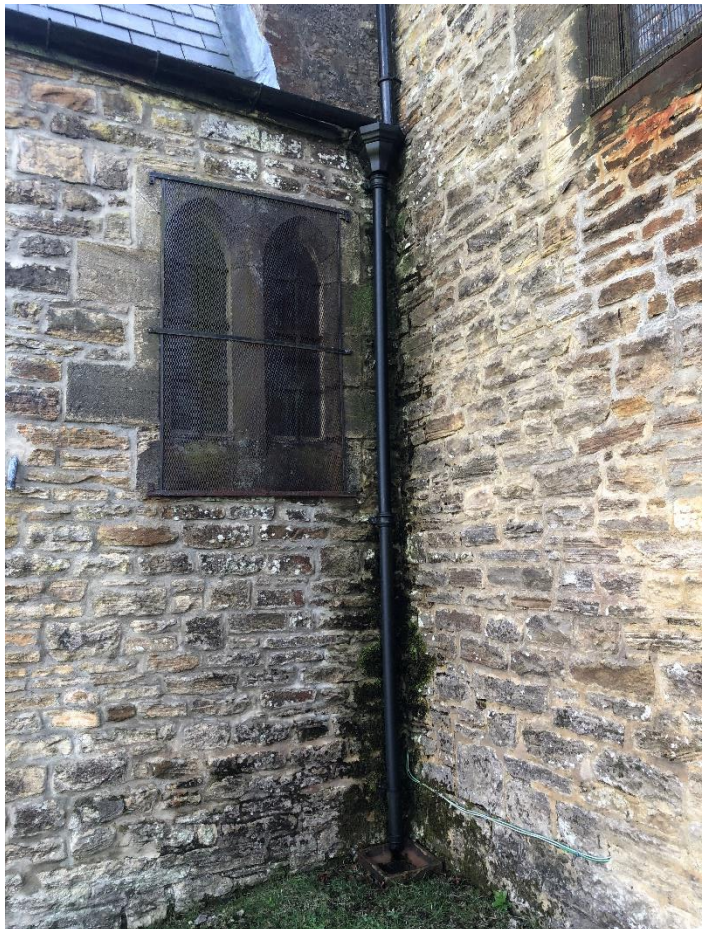
P6 (4801): Vestry (organ loft external downpipe leakage)
