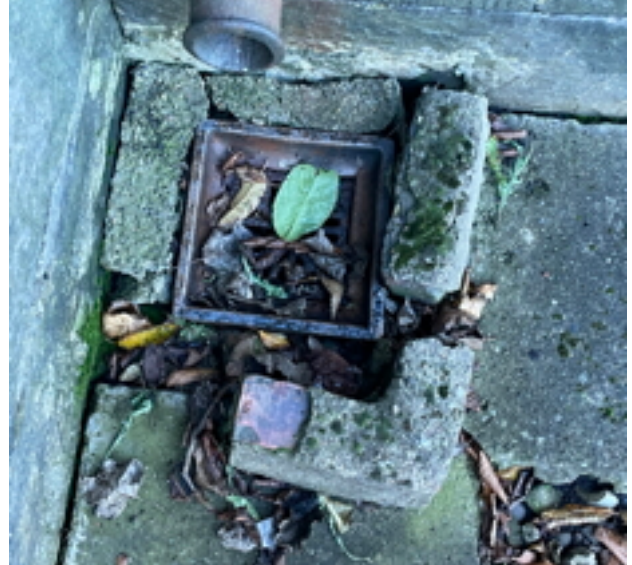
Broken Gully Surround
