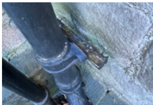
Rotten Wood Block South Elevation
