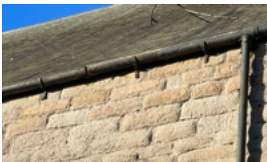
Rusting Gutters South Elevation
