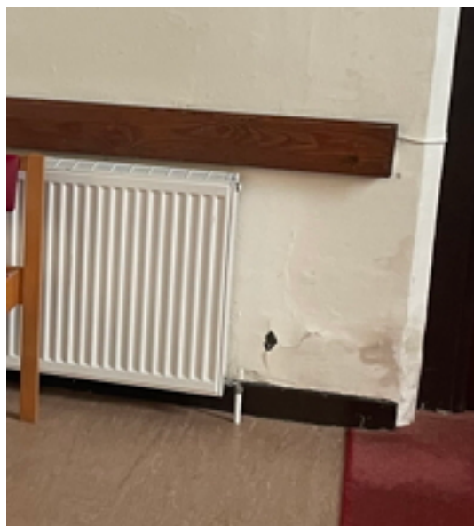
South Wall Rising Damp at South Porch Doorway
