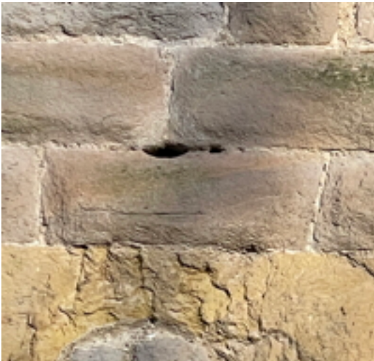
Open Joint to Tower West Elevation
