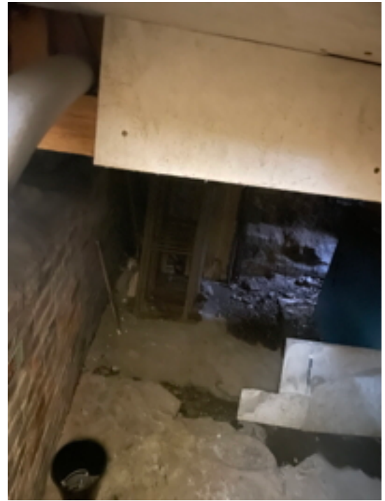
Boiler Room Viewed From Above
