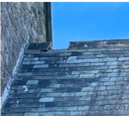
Missing Chancel Ridge Tile
