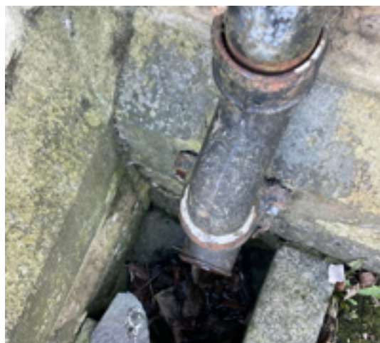
Rusting Rainwater Pipe North Porch
