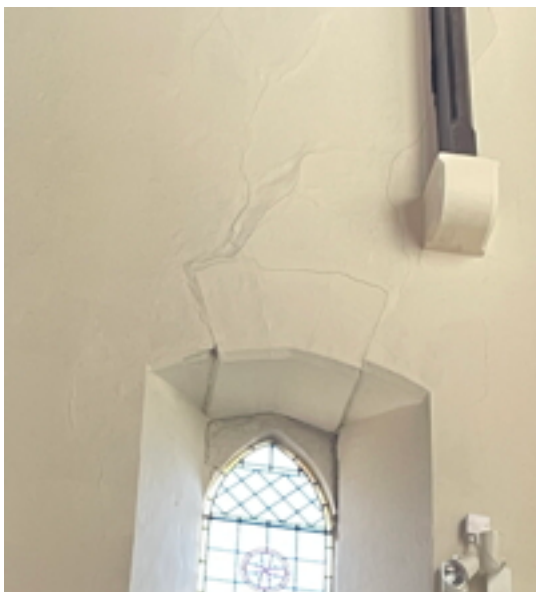
South Wall Cracking Over Window
