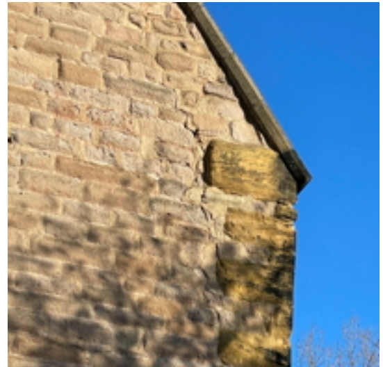
West Gable South Side Cracking
