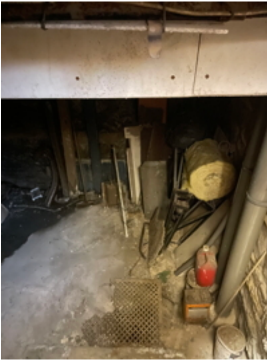
Boiler Room Viewed From Above
