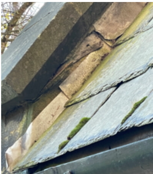
Porch Missing Flashing East Elevation
