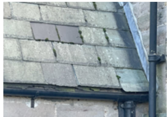
Non-Matching Repairs to Porch
