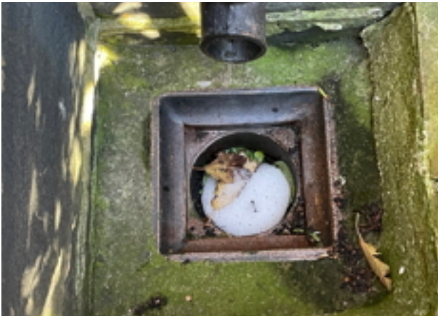
Missing Gully Grating
