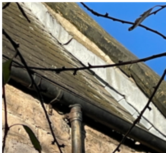
Missing Aligned Copings and Flashing Nave East End South Elevation
