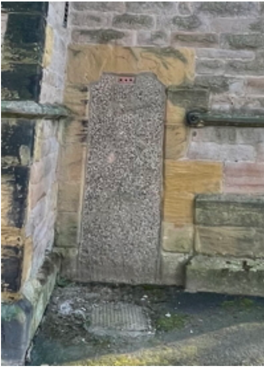
Blocked Tower Door North Elevation
