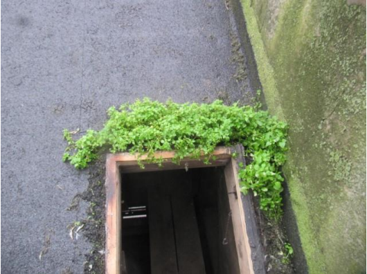
Vegetation growth around the tower roof hatch
