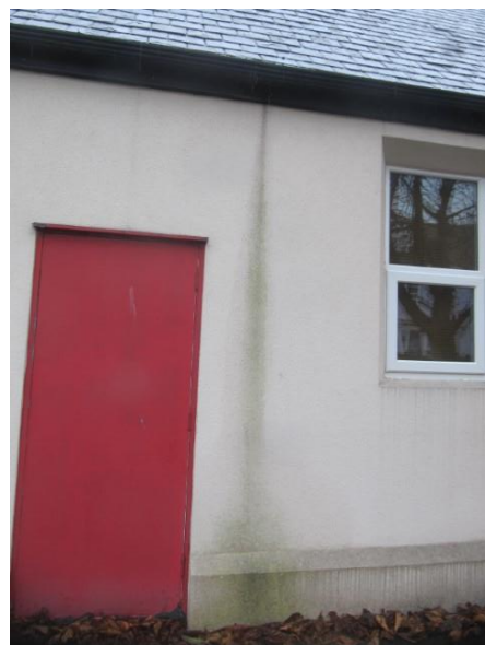
Damp staining under the leaking gutter
