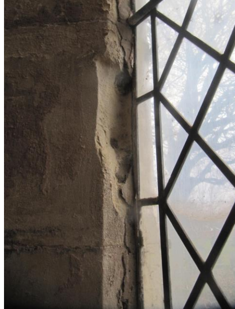
Failing stonework to reveal of Nave window
