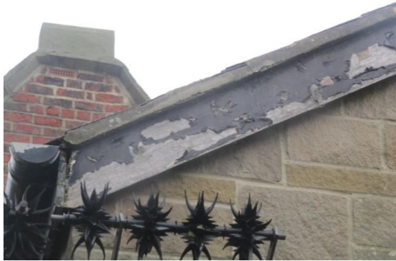
Failing paintwork to East wall of the Hall
