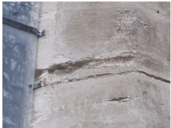
Mortar repair starting to weather to the South Elevation of the Nave
