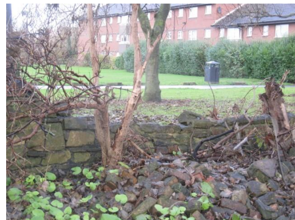
Fallen sections of the Northern boundary wall
