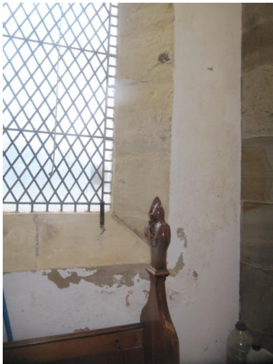
Dampness, salts and failing paint to the West wall in the base of the tower
