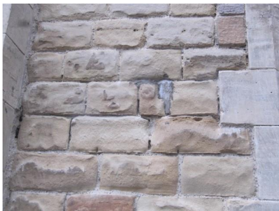
Hungry/Open joints to the South Elevation Of the Nave
