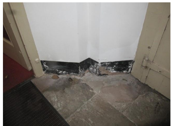
Damage to painted skirting in the same area
