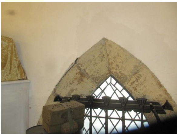
Cracking over the North Gallery window head
