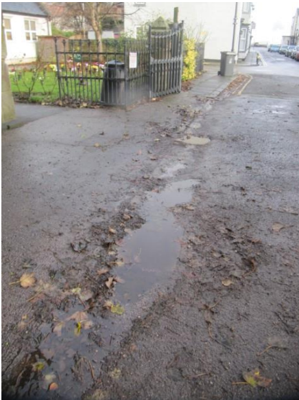
Potholes and ponding to the access road adjacent to the footpath
