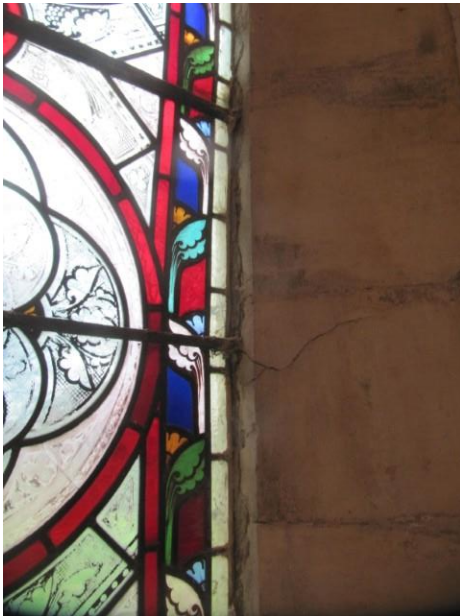
Glazing bars causing damage to masonry to a window reveal in the Nave
