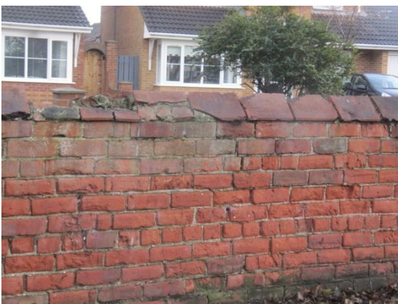
Failing capping, cracking and hungry/open joints to the boundary wall
