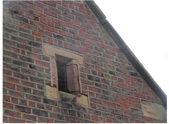
Open joints to the water table, cracking/open joints around the vent and weathered stonework to the East gable of the hall
