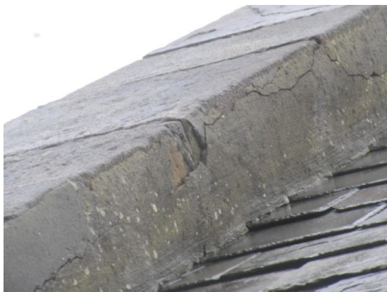
Cracked mortar fillet to the hall roof
