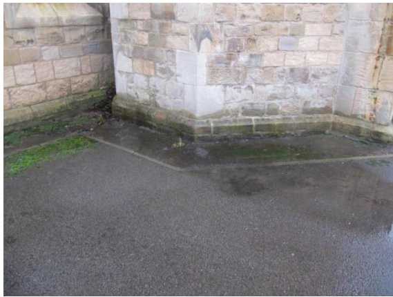
Water ponding to the North of the Tower
