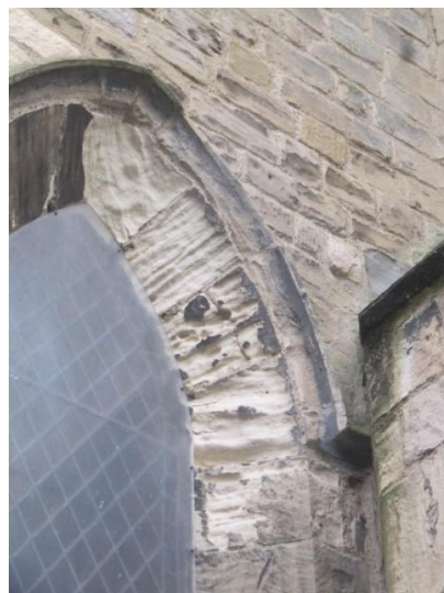
Weathered stonework to the West Nave window (North)
