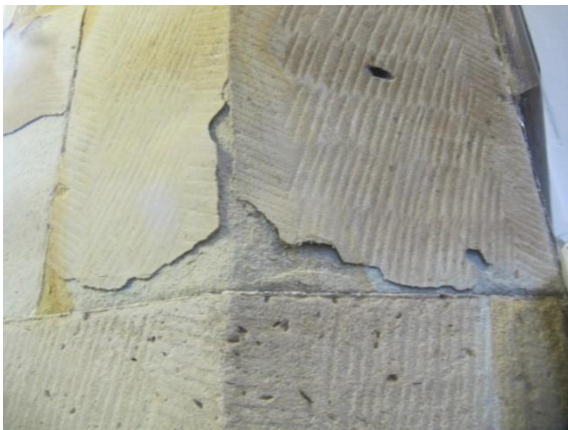
Descaling stonework within the base of the tower
