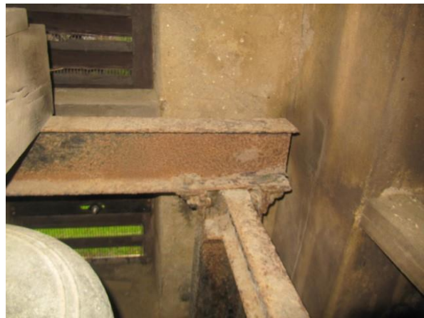
Rusting metal within the bell Chamber
