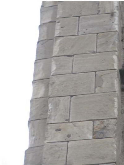
Open/hungry joints to the Northern buttress On the West Elevation of the Tower
