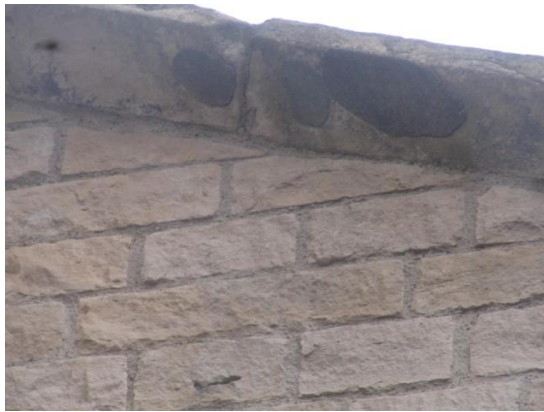
Area of mortar repair to the water tabling to The Nave (West)
