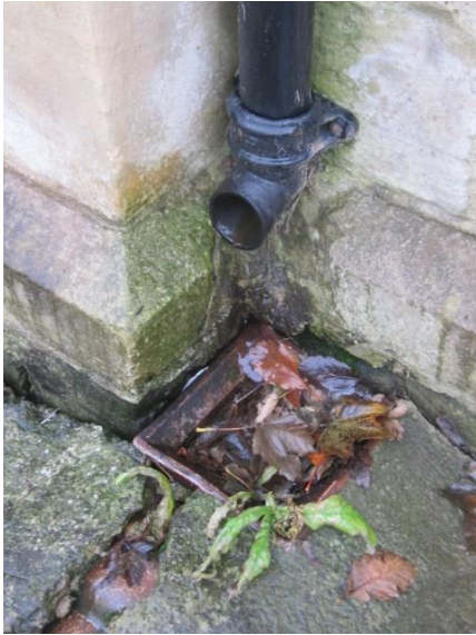
Shoe to the base of the downpipe to the North side of the church needs to be repositioned as adjacent stonework is becoming wet
