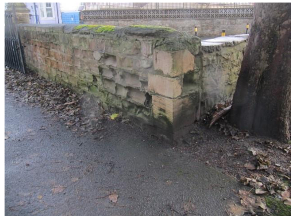
Weathered stone to the side wall near the entrance
