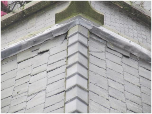
Damaged and slipping slates to the East end of the Nave roof
