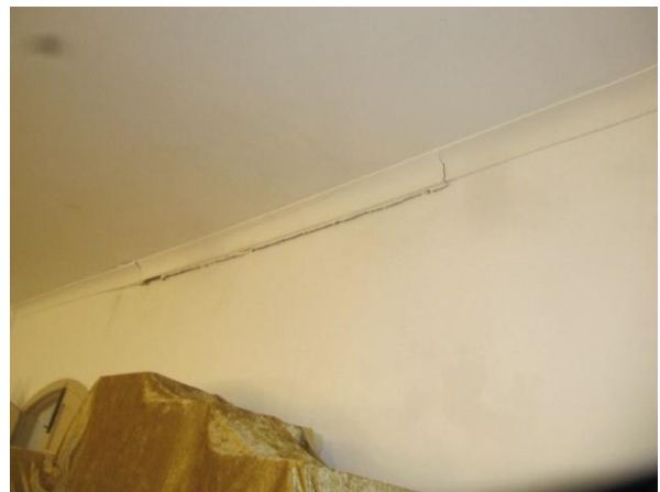
Failing coving to the West wall in the gallery
