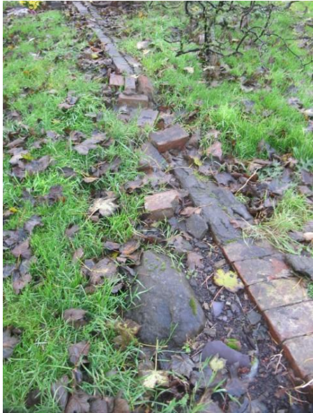
Loose bricks and low wall perpendicular To the Western boundary
