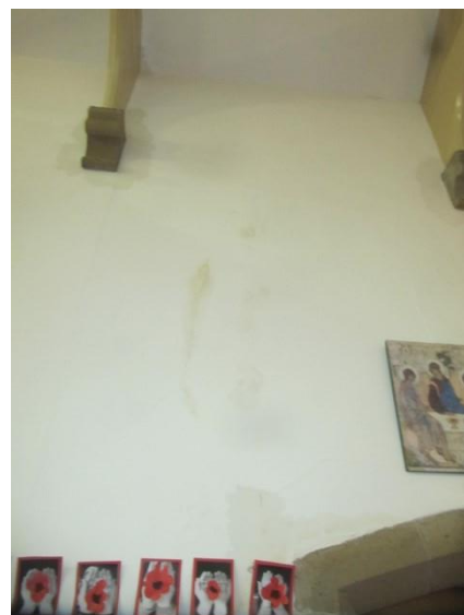
Dampness to the North wall of the Chancel
