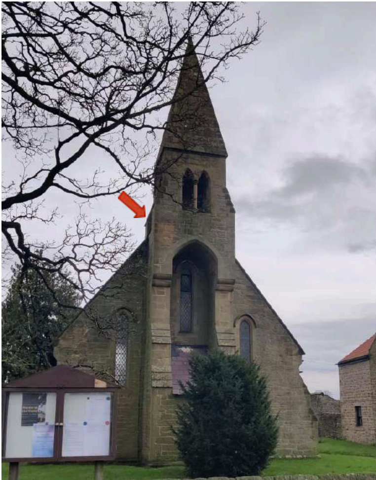
22. View from W: Small area of stonework erosion (arrow) is consistent with condition reported in QIR 2015.
