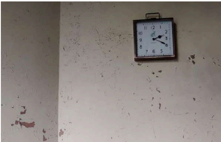
33. Cracking paint seen throughout Nave and Vestry
