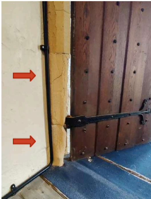
11. Internal door leading from Chancel to Vestry: bottom two stonework courses decaying.
