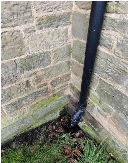
13. Gully at abutment of Vestry & Chancel indicates original ground level. If cracked or not discharging, it could be the source of rising damp.
