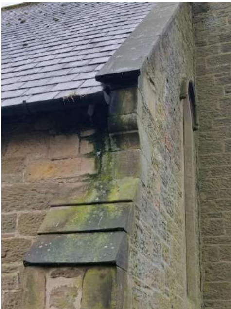
3. NW Nave roof: clean gutter; add lead upstand to roof to prevent water running onto stonework.
