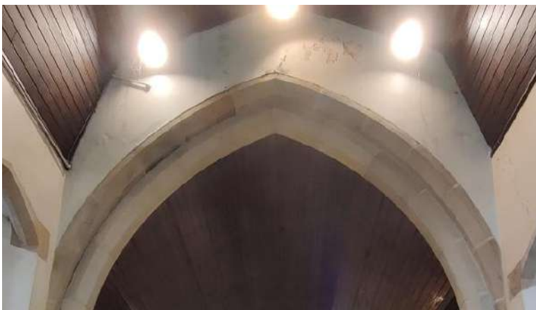
35. Historic water ingress and cracking above Chancel arch.
