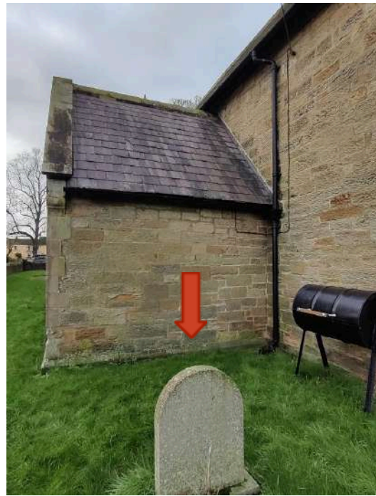
12. Risen ground level obscuring base plinth could contribute to rising damp problem in photo 11.
