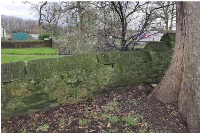
39. NW boundary wall. The cracking and loose copings require periodic re-setting and pointing.
