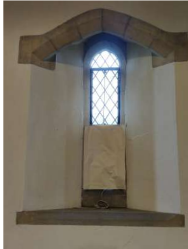
28. Nave N wall: broken leaded light
