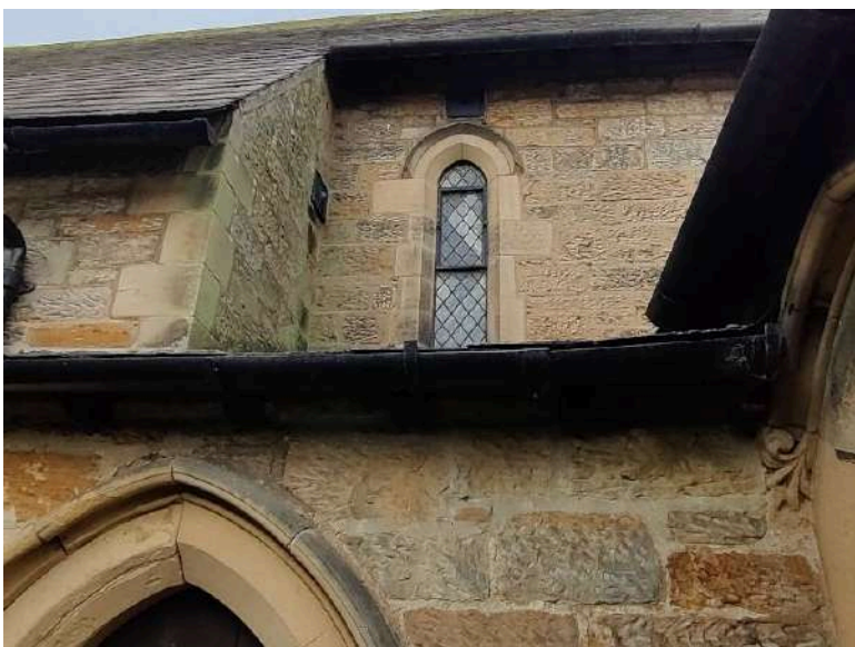
20. Same issue at the SE abutment of the Nave marked by the greening of the sandstone wall.
