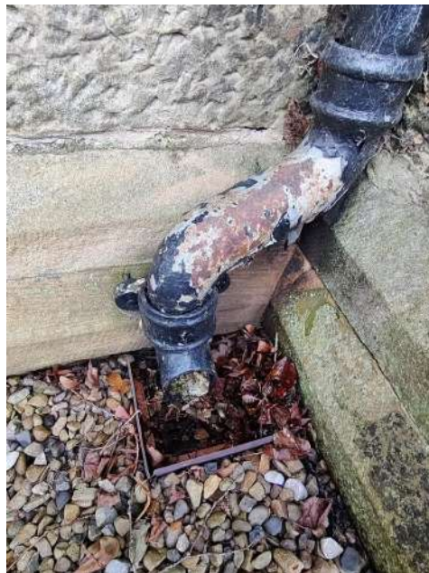
4. Localised need to repaint downpipe.
