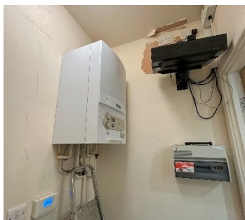
Figure 16 – Boiler and CU
