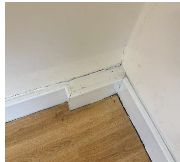
Figure 13 – Hall shrinkage to walls
