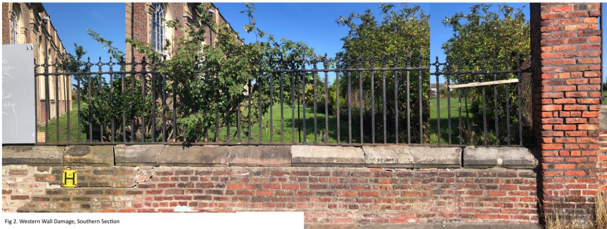
Fig 2. Western Wall Damage, Southern Section
