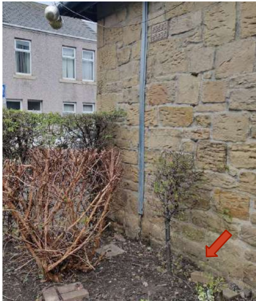
9. Lower ground floor levels at SW (rec. 2.03) ...
