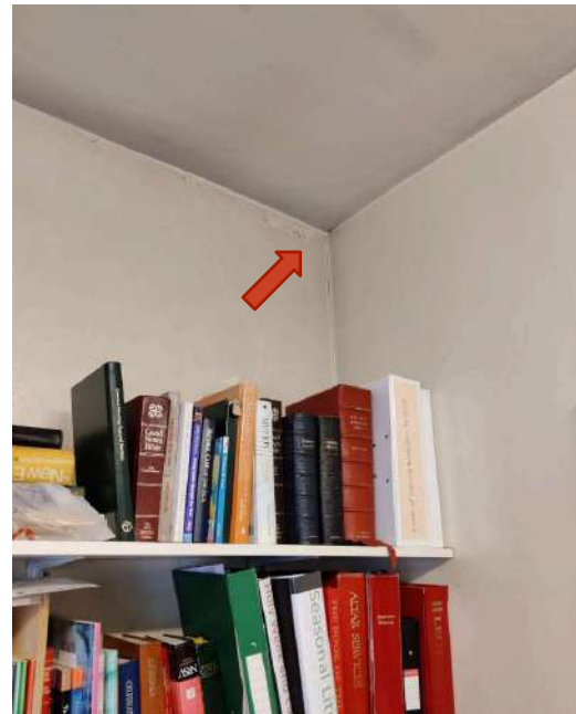
17. Vestry. Monitor cracked plaster to NE (rec. 4.02)
