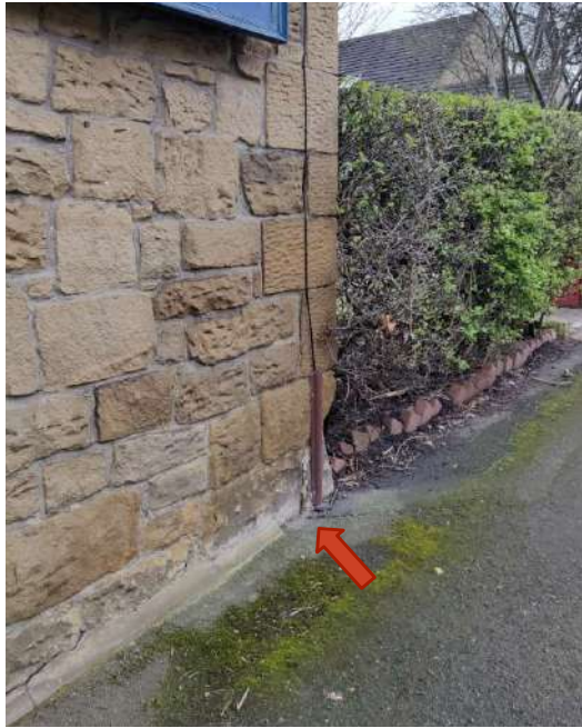
7. Replace missing or broken areas of the mortar fillet to the base of the W elevation (rec. 2.01)
