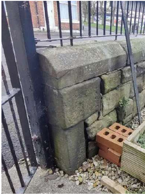
47. North Yard. Dismantle, rebed and repoint loose stonework and quoins (rec 8.02)
