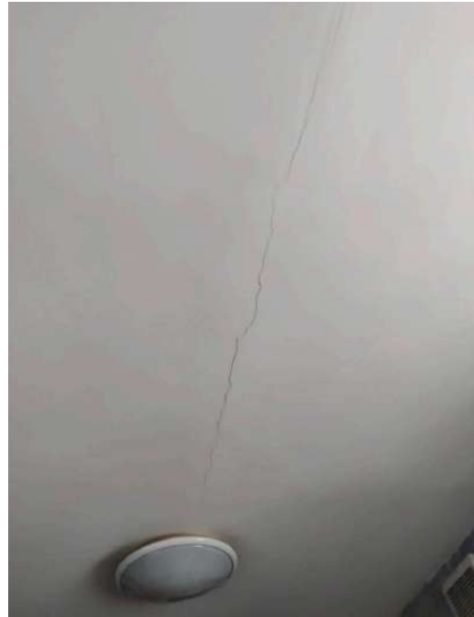
44. Room 1. Monitor ceiling crack (rec 4.12)
