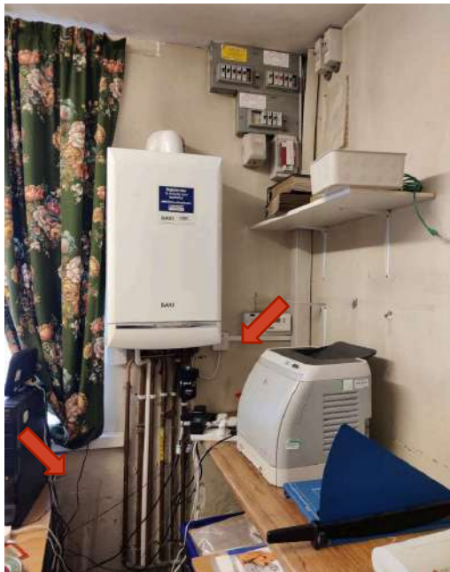
16. Vestry. Consider replacing failing plaster to W wall. (rec. 4.03)
