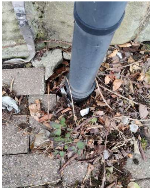
6. Example of blocked gully to the West requiring clearing (rec. 1.03)
