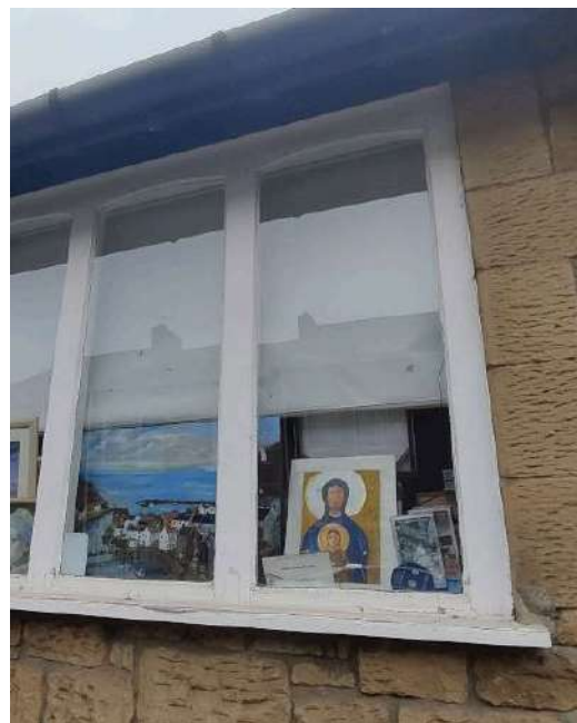
14. Consider redecorating window joinery to E and W elevations (rec. 3.02)
