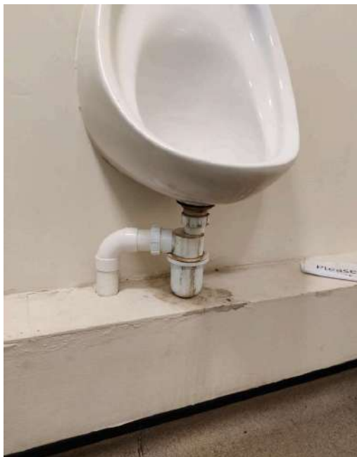
31. Fix leaking urinal & redecorate (rec. 4.07)
