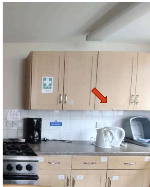
26. Consider replacing peeling veneer (rec. 4.05)
