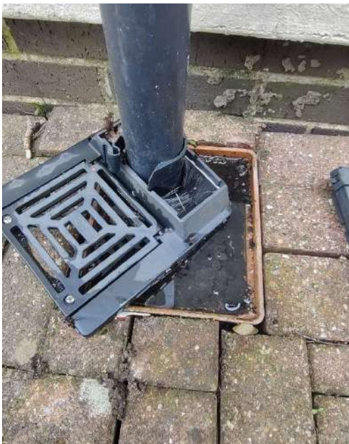
5. Example of blocked gully to the South requiring clearing (rec. 1.03)
