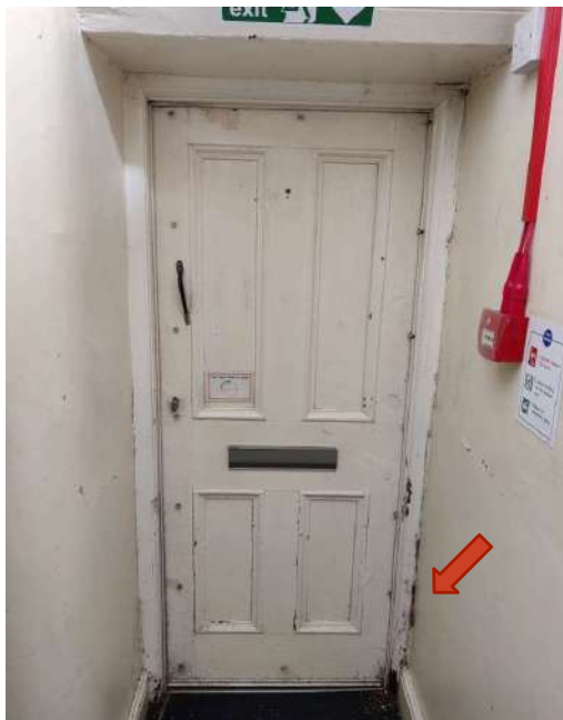
38. North fire exit door. Repair decayed base of frame. Redecorate door & frame. (rec 4.10)
