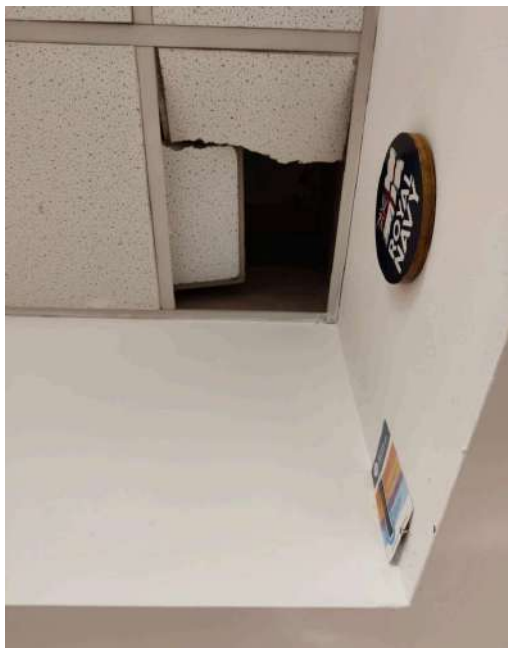
41. Replace broken ceiling tile (rec 4.11)
