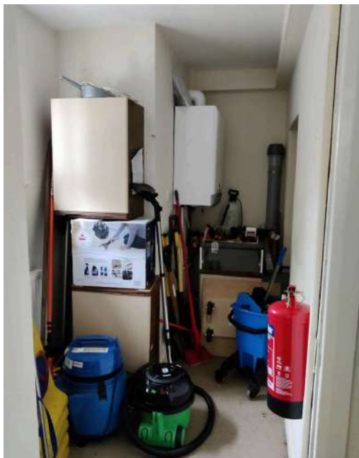
25. Storage room near kitchen with gas boiler 1
