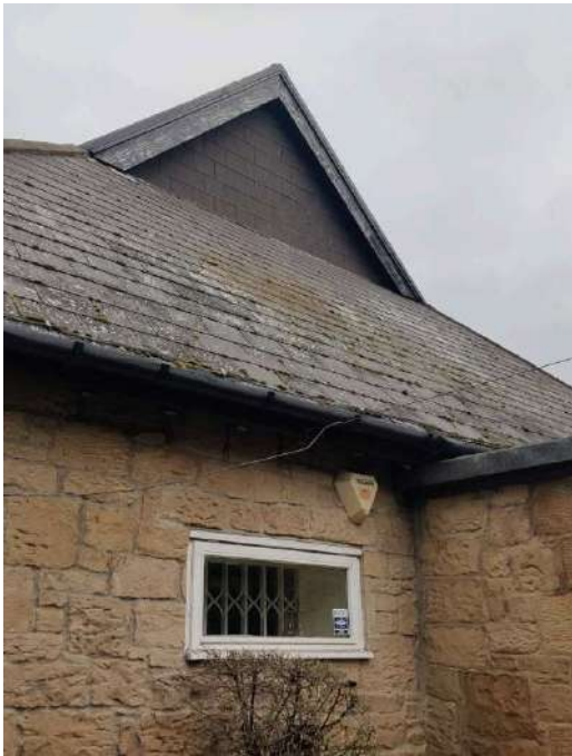
5. Timber barge boards to south gable require redecoration (recommendation 1.01)
