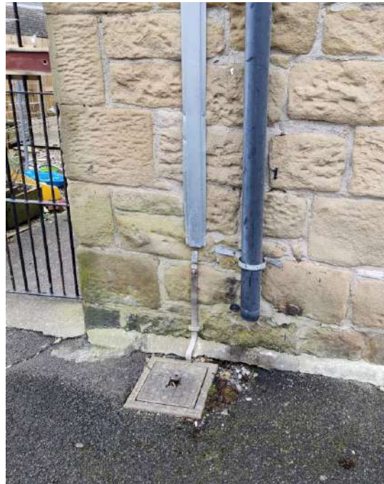
6. The missing shoe to the northwestern downpipe should be replaced (rec. 1.02)
