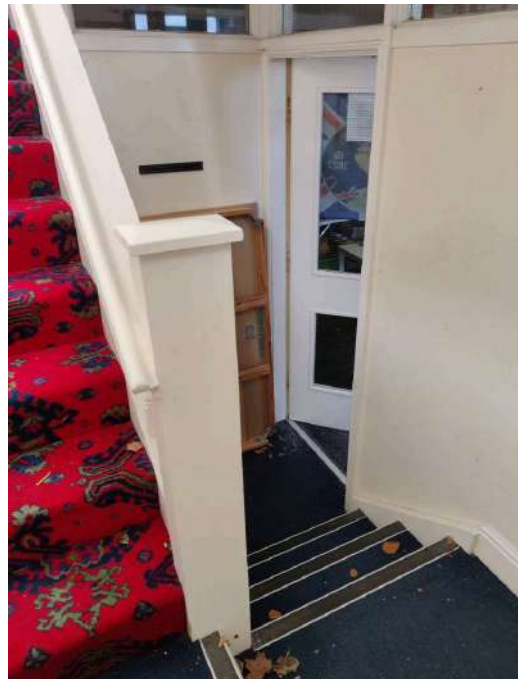
37. Partition at base of stairs. Review need for fire upgrade if unit is let (rec. 6.02).
