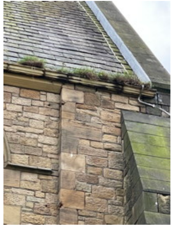
North Nave Blocked Gutter
