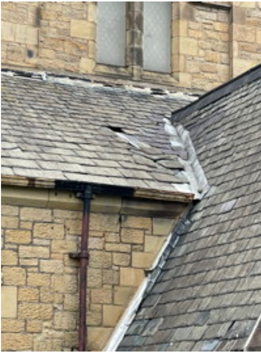
South Aisle Missing Flashings and Slates
