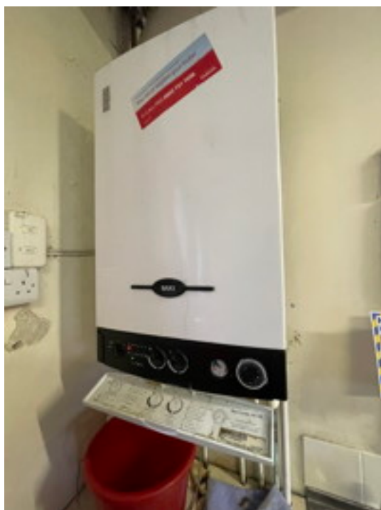
Vestry Store Boiler
