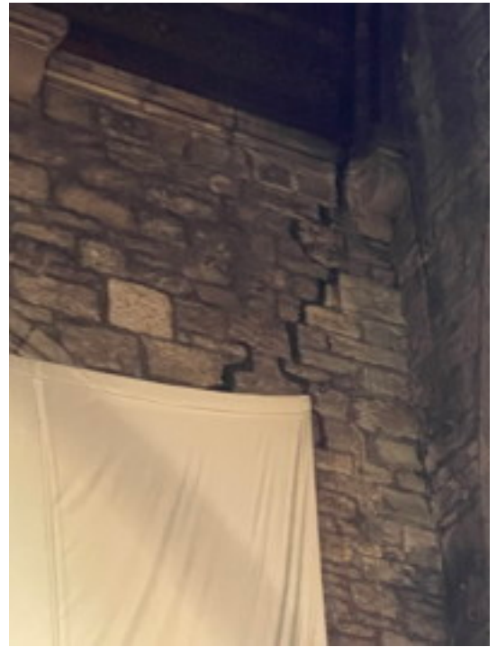
Cracking to Chancel South Elevation
