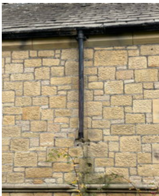
South Aisle Missing Rainwater
