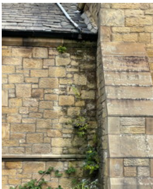
South Aisle Missing Rainwater
