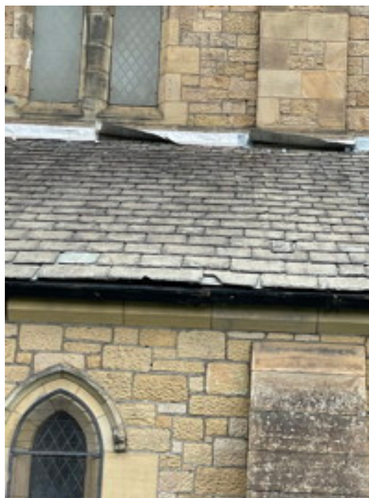
South Aisle Displaced Flashings
