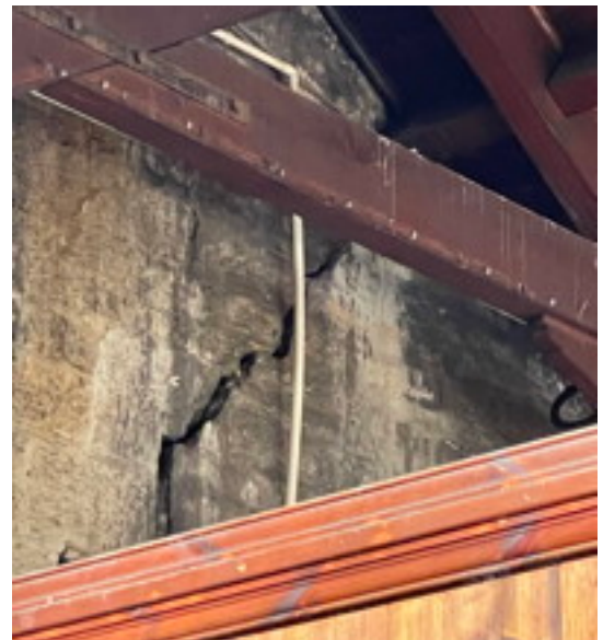
West Wall Cracking Over Kitchen
