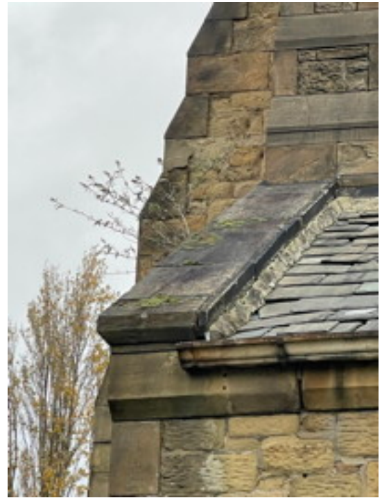
South Porch Open Joint
