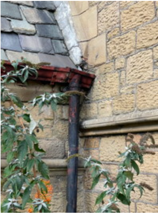
South Porch Misaligned Gutter
