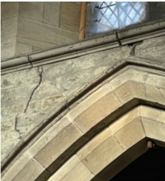
Nave Cracking to West End
