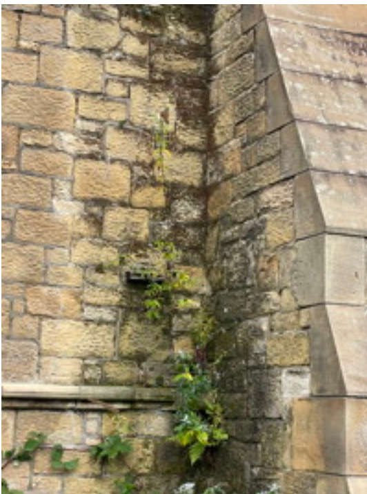
Plant Growth and Missing Rainwater Pipe Location
