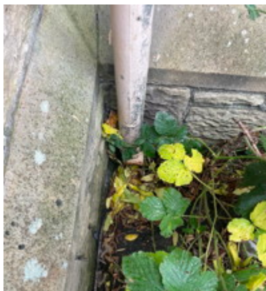
Typical Gully blocked with vegetation
