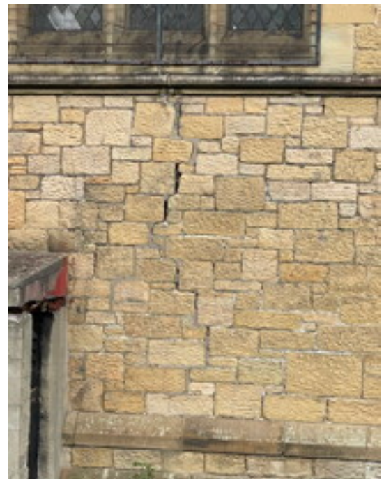
Cracking to Organ Chamber South Elevation
