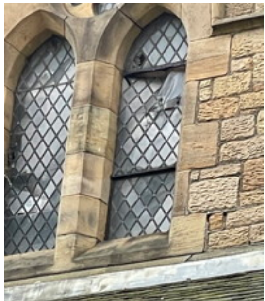
Typical Vandalised North Elevation Clerestory Window
