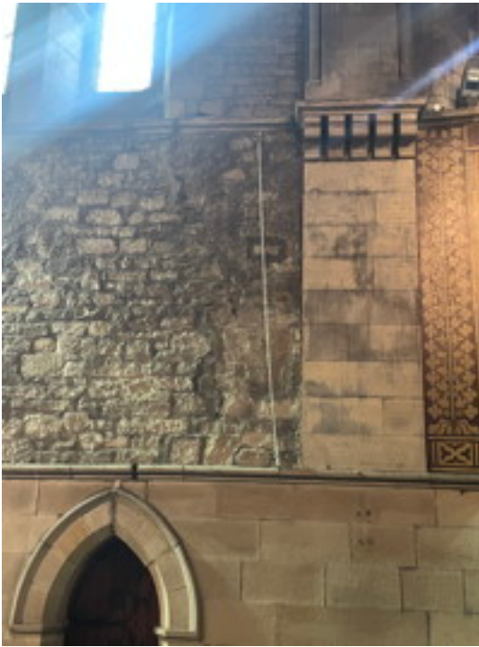
Cracking to Chancel North Elevation
