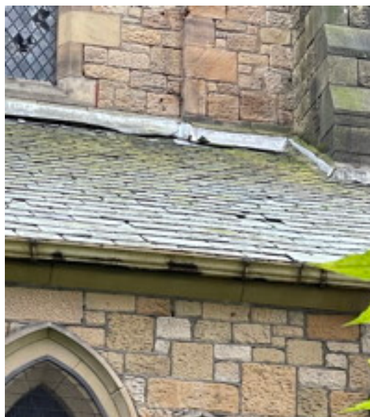
North Aisle Displaced Flashings
