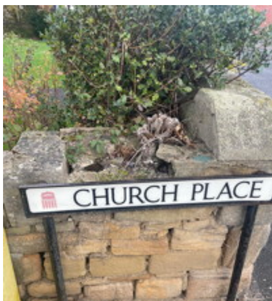
Tree Damage South East Corner
