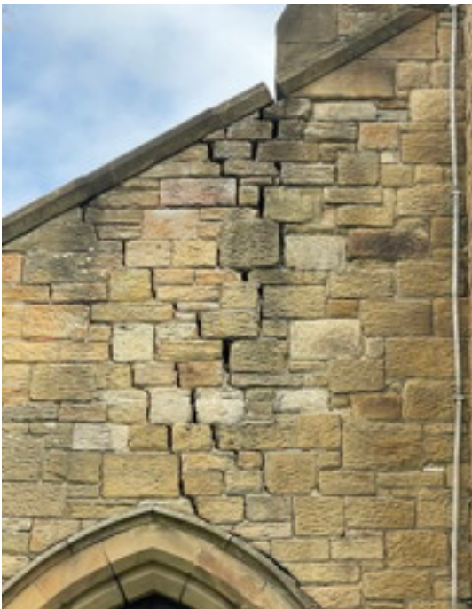
Severe Displacement Over Door to West Elevation North Side
