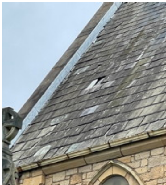
Nave South Elevation Missing Slate
