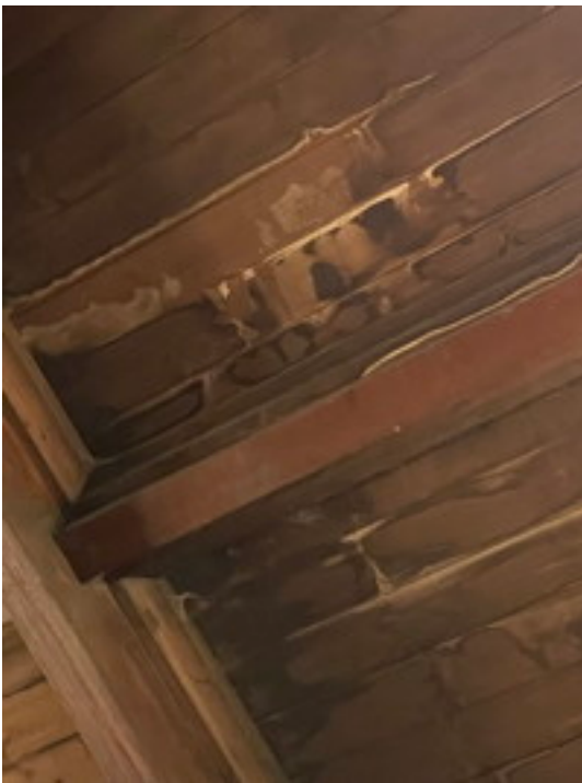
Staining to South Aisle Ceiling
