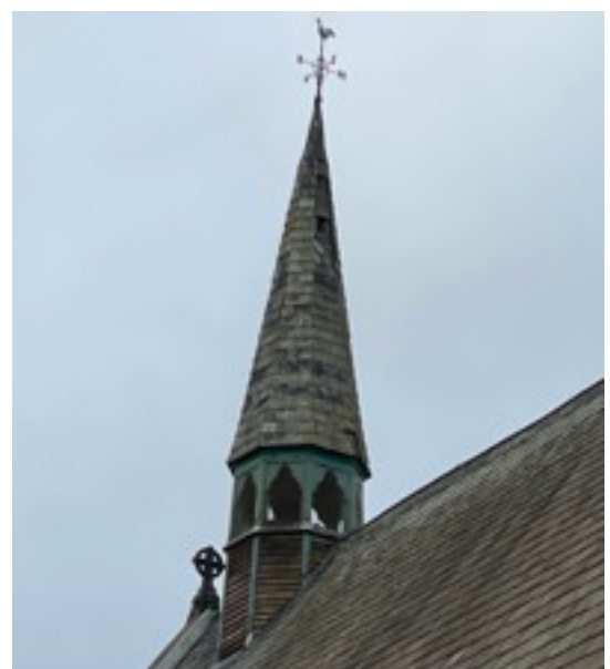
Flèche Missing Slates
