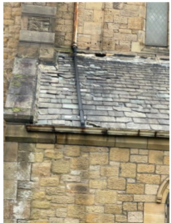
South Aisle Many Displaced Slates and Missing Flashings
