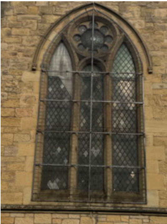
Organ Chamber Missing Glazing
