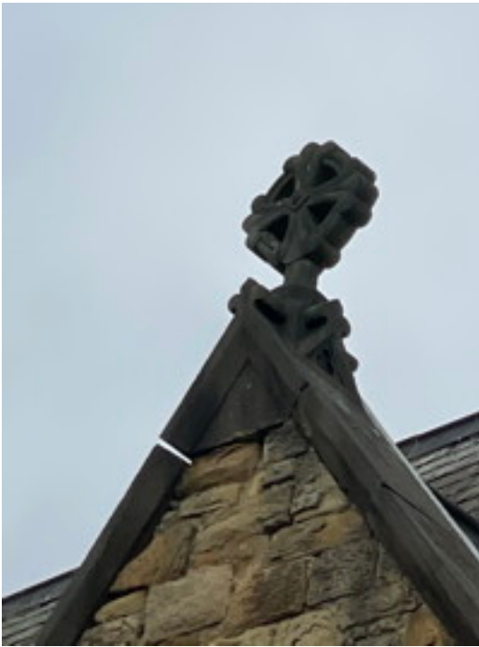
South Porch Open Joint
