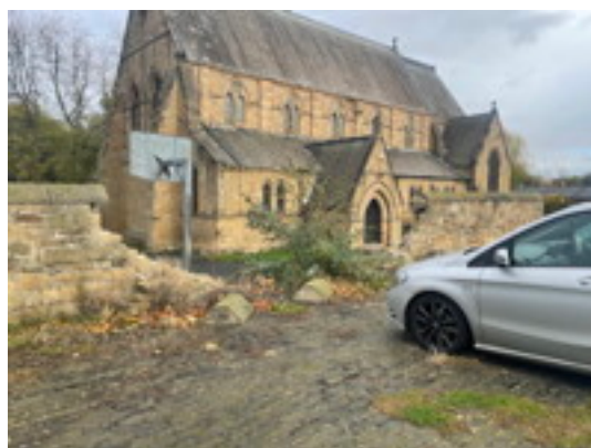
Collapsed South Boundary Wall
