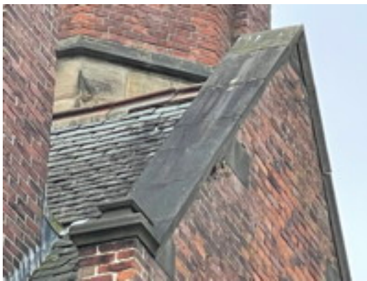
Fern Below North Gable Parapet
