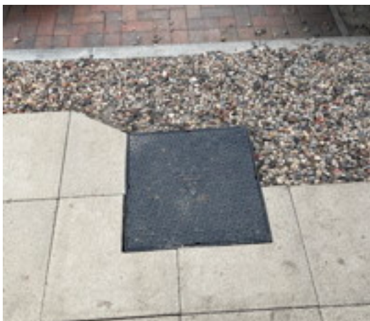
Larger Inspection Chamber
