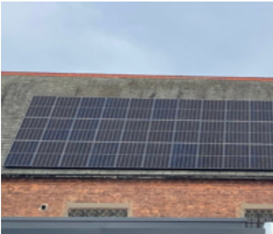
South Elevation Misaligned Gutter
