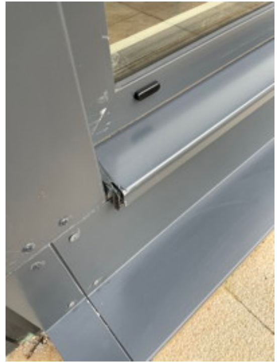
Damaged End cap
