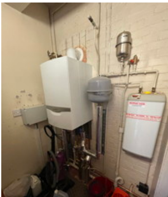
First Floor Boiler Room
