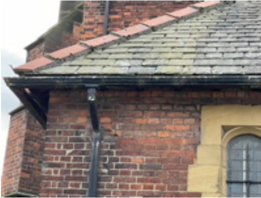
North Elevation Gutters and Rainwater Pipes in Need of Decoration
