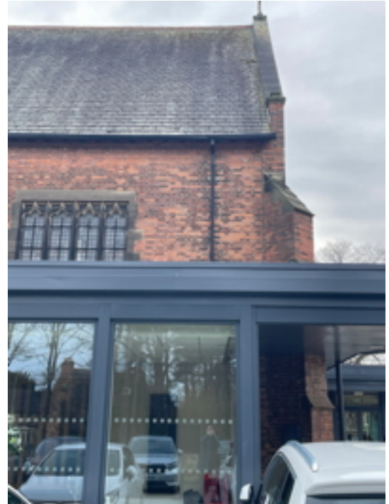
North Elevation Rainwater Pipe Discharging over Flat Roof
