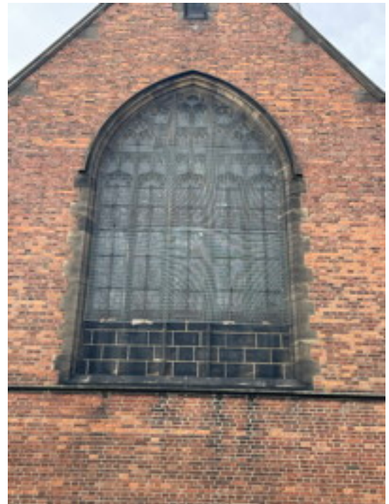
East Window Metal Grilles
