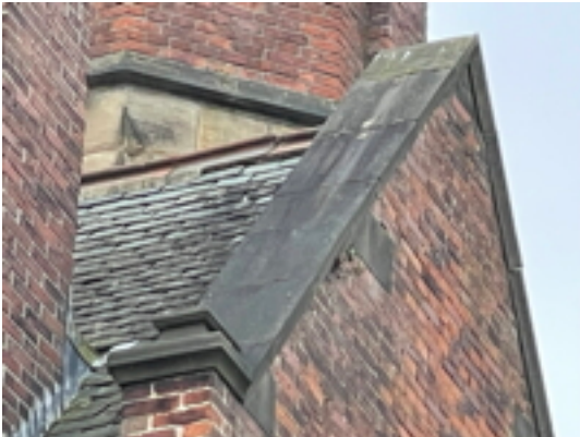
Missing Ridge Pointing North Gable East Elevation
