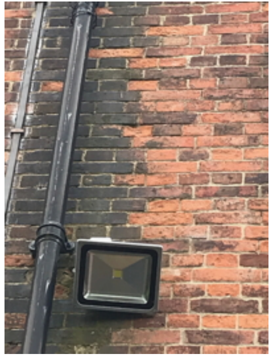
Erosion of brick faces to North
