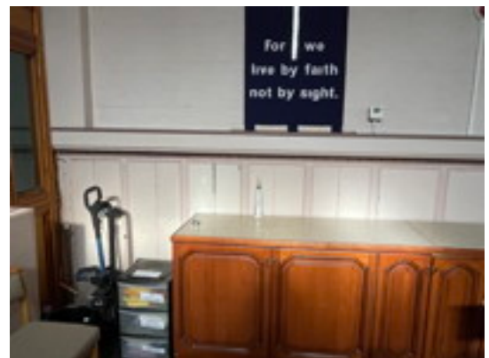
Typical Shrinkage Cracking to Panelling
