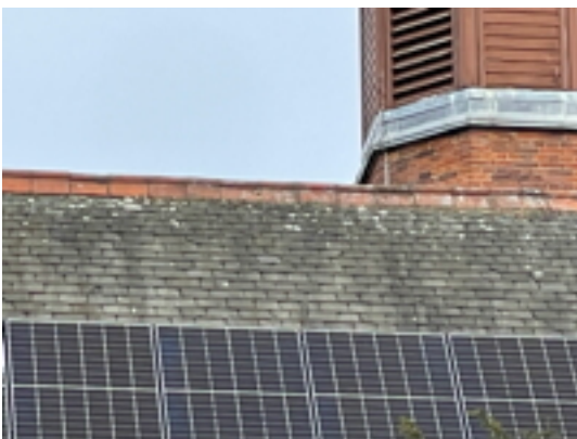
Broken Slates South Elevation
