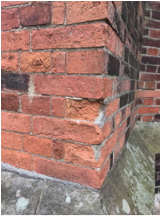
Erosion of brick faces to buttress
