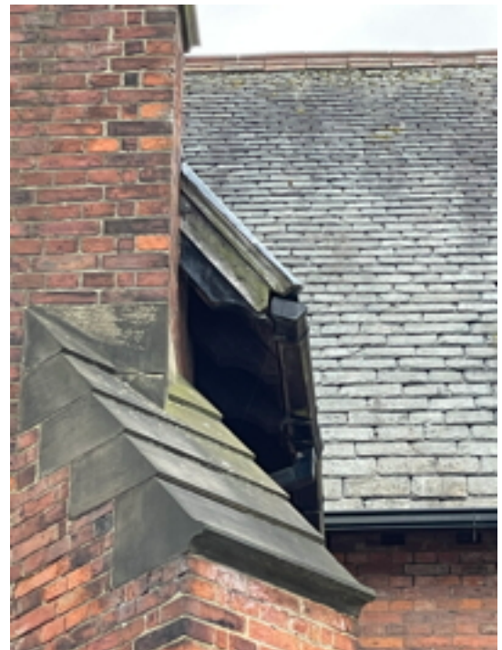
Misaligned West Elevation Gutter
