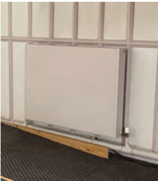
Typical Nave Radiator
