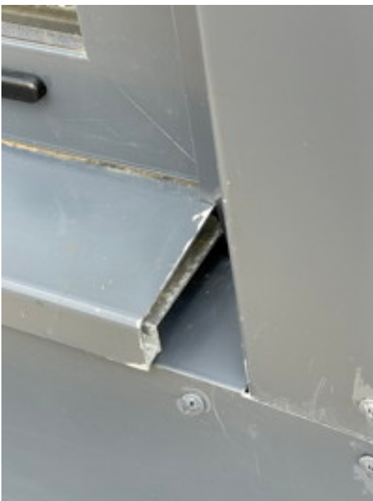
Missing End cap
