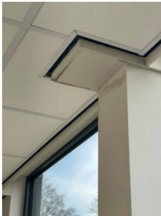
Multi-Purpose Room Water Damaged Ceiling
