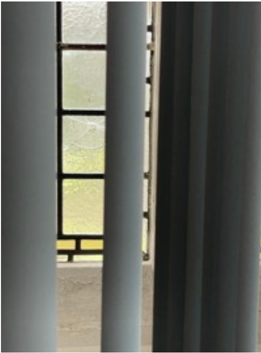
Broken Vestry Window Pane
