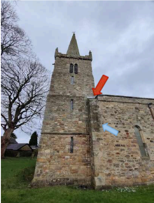
40. Tower S elevation. Exposed wall head at W end of Nave (red arrow) and water ingress (blue)
