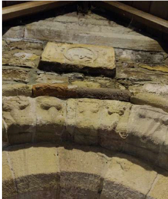
4. The salt efflorescence above the north door is similar to that reported in QIR 2015.
