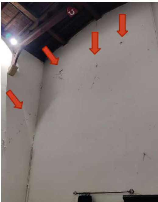
15. Wide-spread failing plaster at high-level at the West end of the Nave (arrows)
