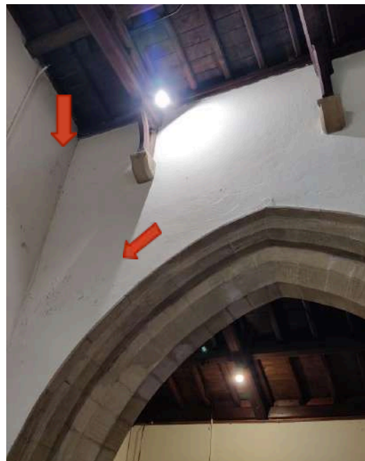
16. Failing plaster at the Northwest abutment of the Nave to the North Aisle (arrows)
