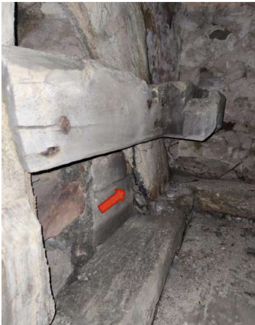
63. Wetness & decay to historic bellframe (arrow)
