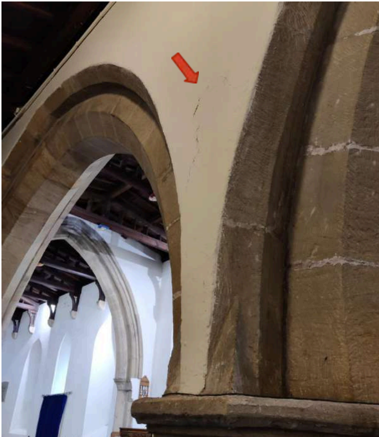
12. Failing plaster at base of arch between North Aisle and Nave (arrow)
