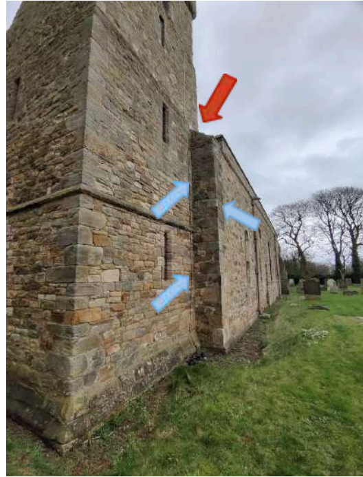
41. Nave W abutment with exposed wall head (red arrow) and signs of water ingress (blue)
