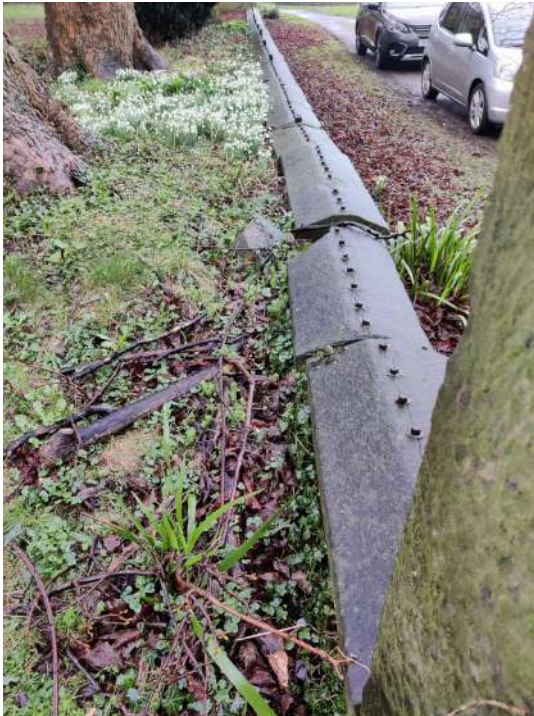
68. N boundary wall disturbed by tree roots
