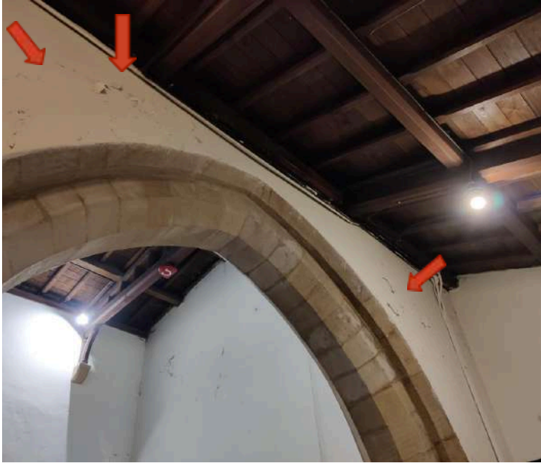
11. Large area of failing plaster at Southwest abutment of North Aisle to Nave (arrows)
