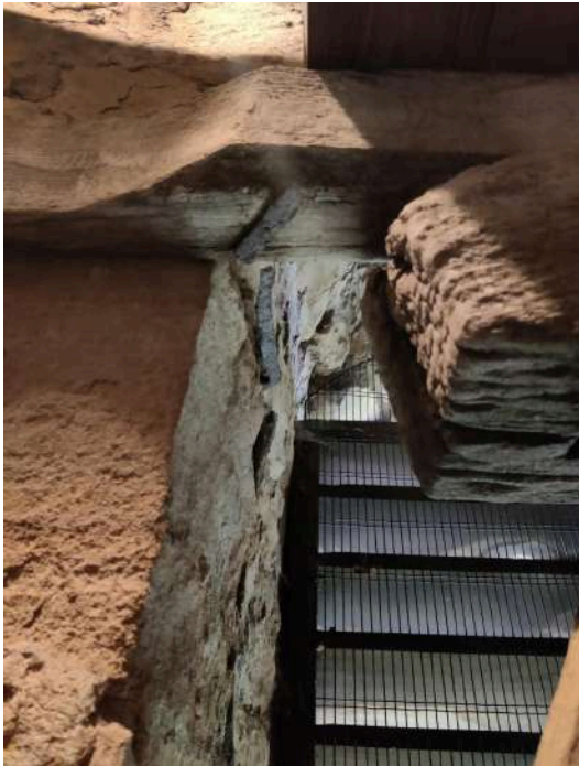
61. Tower top floor, netted louvred openings and redundant timber bell frame, which is wet to the touch and decaying at its base.
