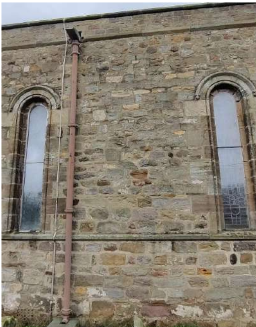
42. S elevation of Nave showing blistering paint internally near location of downpipe. No external defect is visible. Roof outlet should be looked at.
