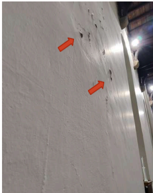
20. Blistering of paint on South wall of Nave, likely connected to external rainwater pipe or outlet
