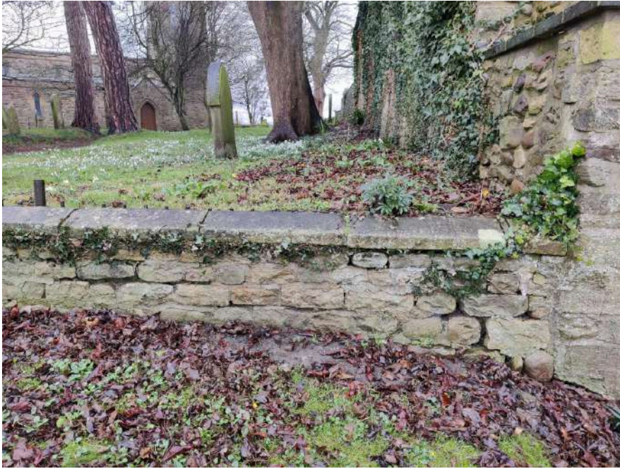
67. E end of N boundary wall - Ivy should be cut, let to die and then carefully removed. The wall and coping stones should be repointed.
