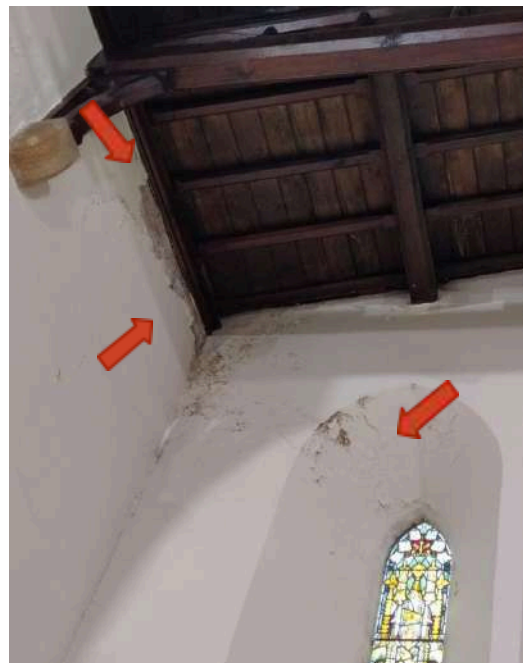
24. Past water damage to E ceiling abutment of Chancel, reported as repaired
