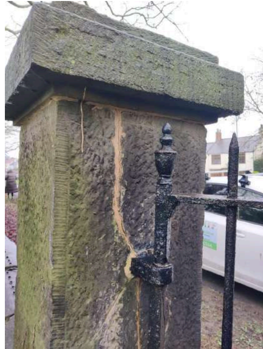
69. Crack requires repointing or complete treatment of rusting hinge end.
