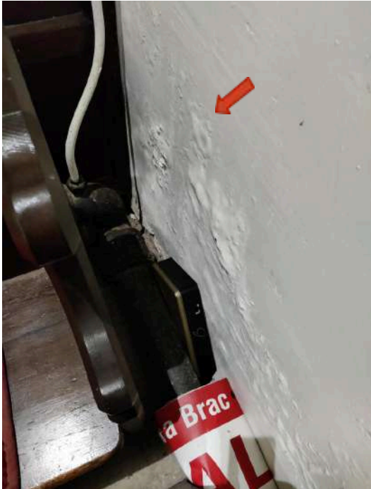
17. Localised blistering plaster at low level at the West end of the Nave
