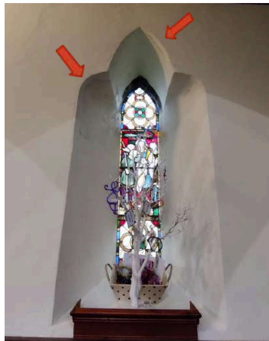
10. Wide-spread racking plaster at window abutments in North Aisle (arrows)
