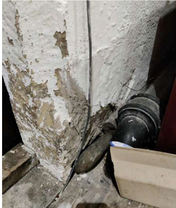
18. Localised failing plaster at low level at the West end between Nave and North Aisle
