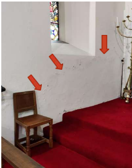
23. Signs of rising damp to N wall of Chancel, same as mentioned in QIR 2015
