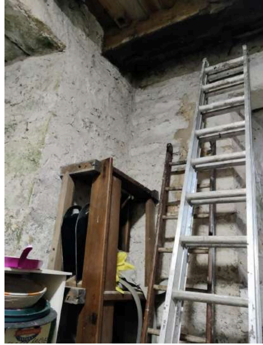
58. Tower ground floor is used for storage. The mouldy smell reported in QIR 2015 is not prominent.
