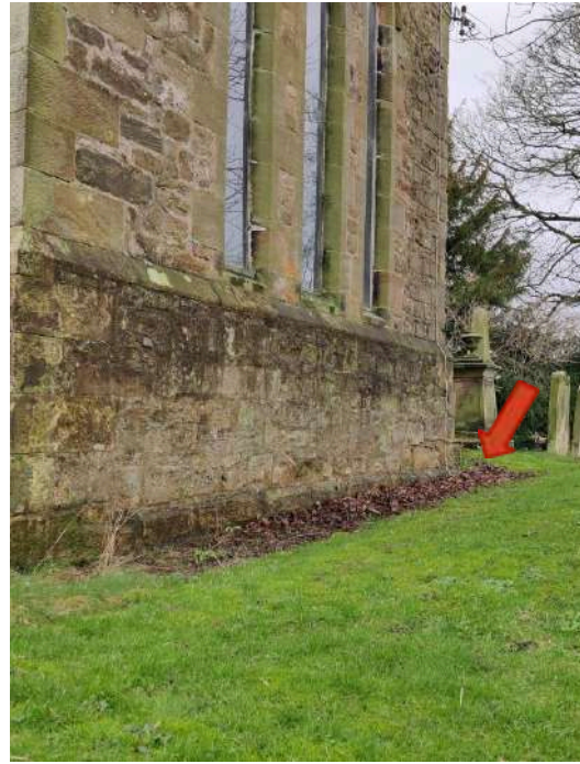
45. Consider reducing local ground to below plinth level should damp problems persist
