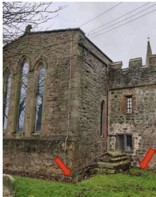
47. As above, consider reducing ground should damp problems persist (arrows)
