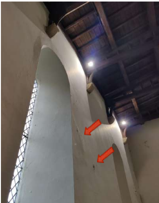
19. Blistering of paint on South wall of Nave
