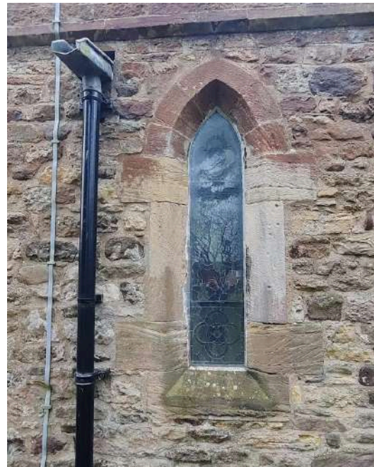
50. North Aisle window. Internal plaster is cracking. The external stonework is generally wet but there is no visible external defect.
