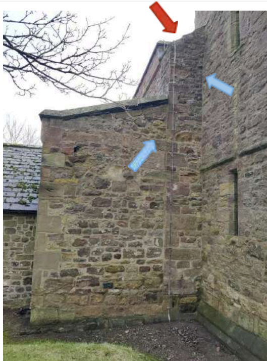
36. Lower tower N elevation. Exposed wall head of Nave (red arrow) and water ingress (blue)
