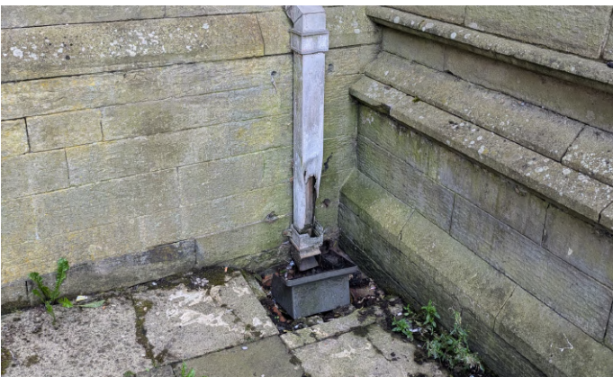
Damage to downpipe on north elevation.
