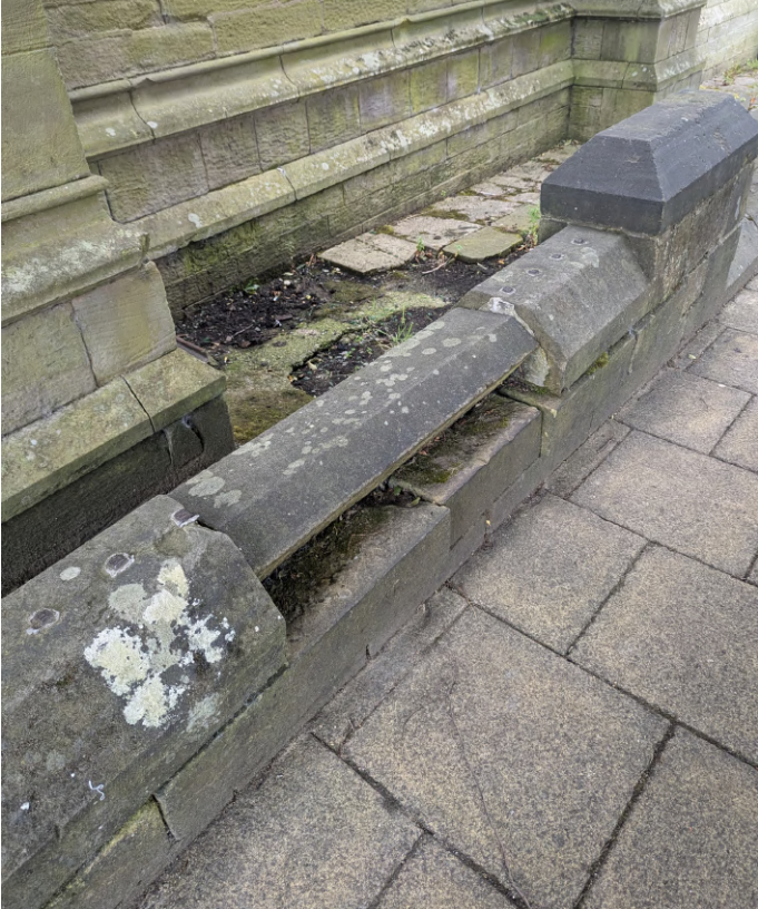
Railings missing from western end of north boundary wall. Areas behind boundary walls to be cleared regularly and kept tidy. Dislodged coping stone required re-bedding.
