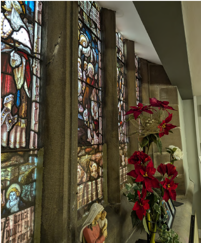
Re-pointing and minor repairs to glazing required to west window.
