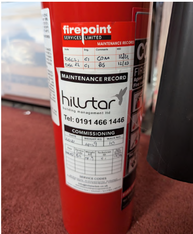
Fire extinguisher in choir vestry.
