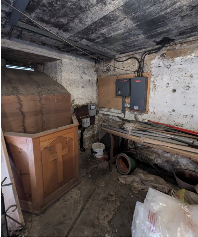
Services within basement at west end of church
