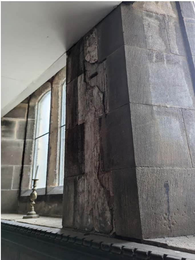
Issues with water ingress at choir vestry due to blocked gutters. Requires replastering after overhaul of rainwater goods.
