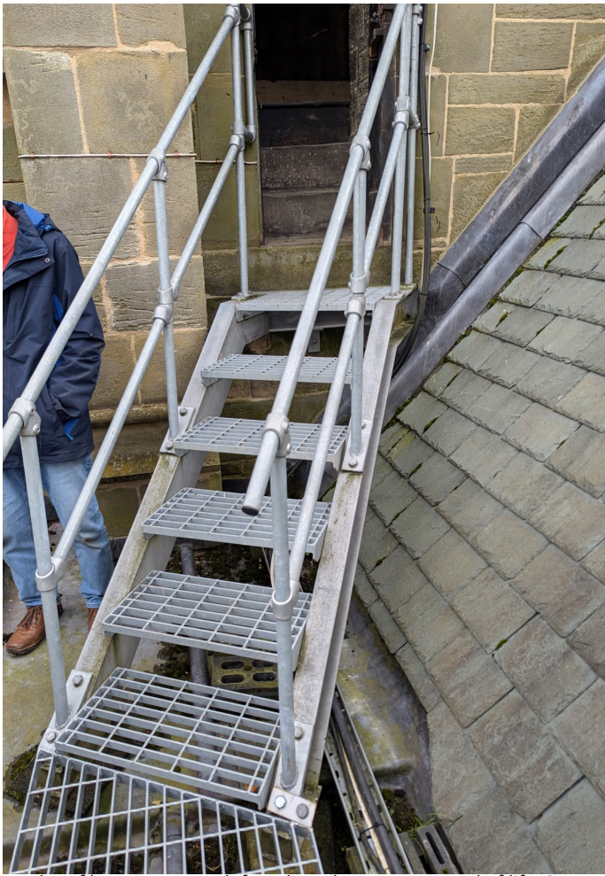
Lead roof between organ loft and north transept at end of life. Steps unsteady. Vegetation build up.
