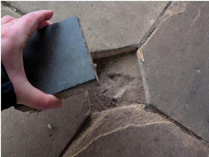
Loose tiles in ambulatory.
