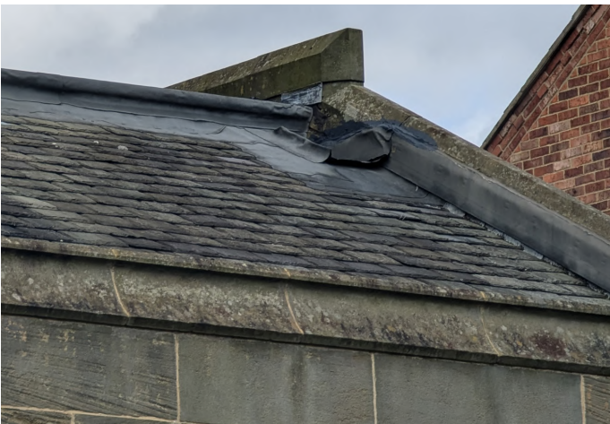
Areas on south chancel roof where flashings have been peeled back by thieves looking for lead
