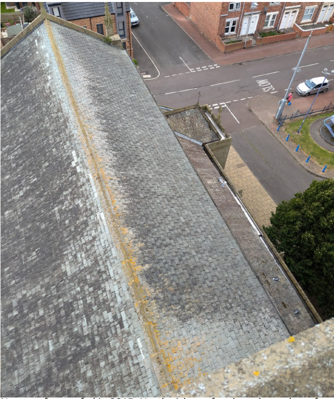
Nave roof re-roofed in 2015. North aisle roof and north porch roof beyond.
