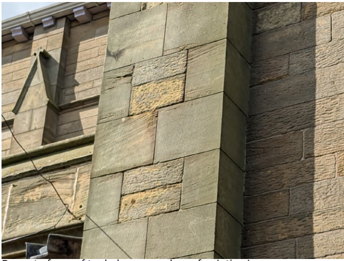
Decay to faces of tooled masonry, loss of pointing in some areas.
