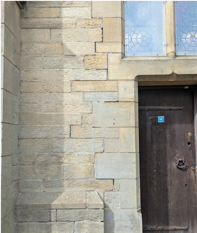
Movement to masonry on left side of south garden door. Now historic. Requires repointing.
