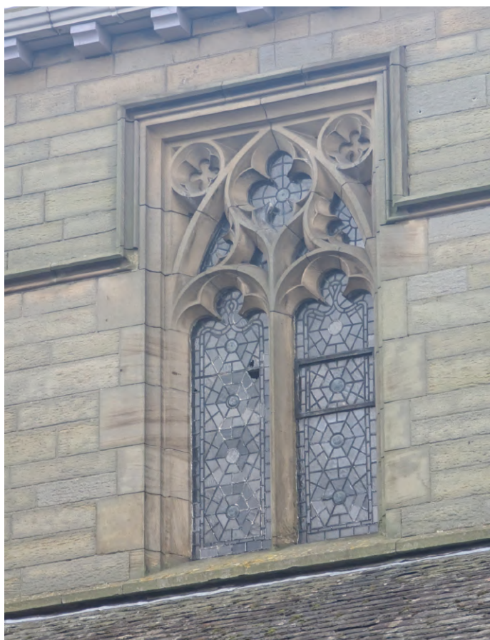
Vandalism to clerestory window on north side of church.
