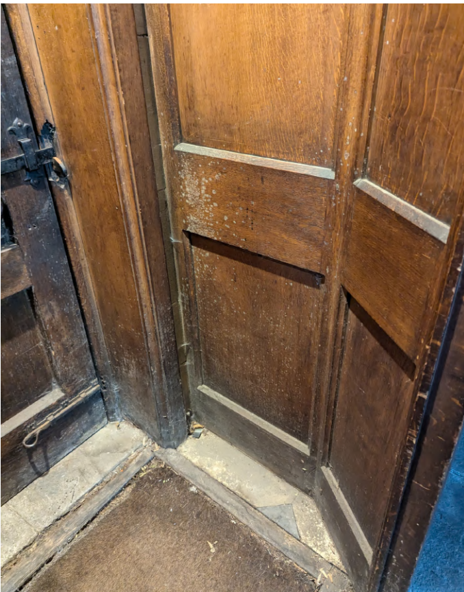
Mould to inside of north aisle draught porch, on both timber and mat. Poor ventilation still a problem.
