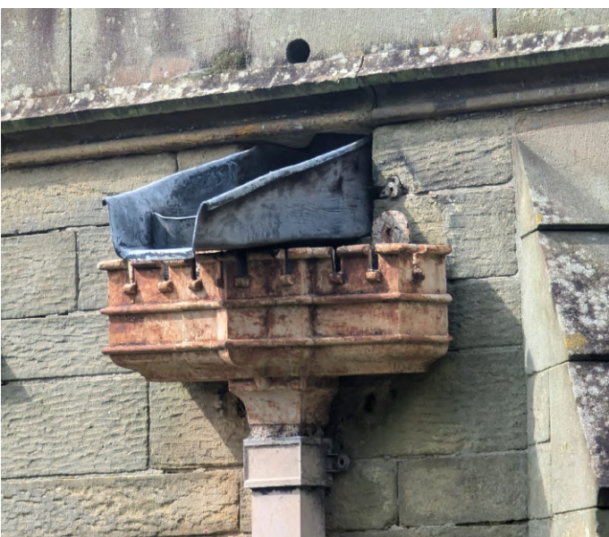
Hopper and downpipe to south retro-chancel elevation. Requires refurbishment.
