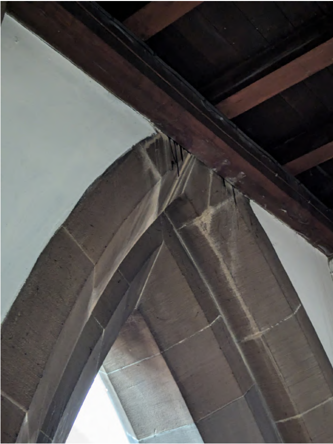
Water staining over window in Angel Loft/east ambulatory area.
