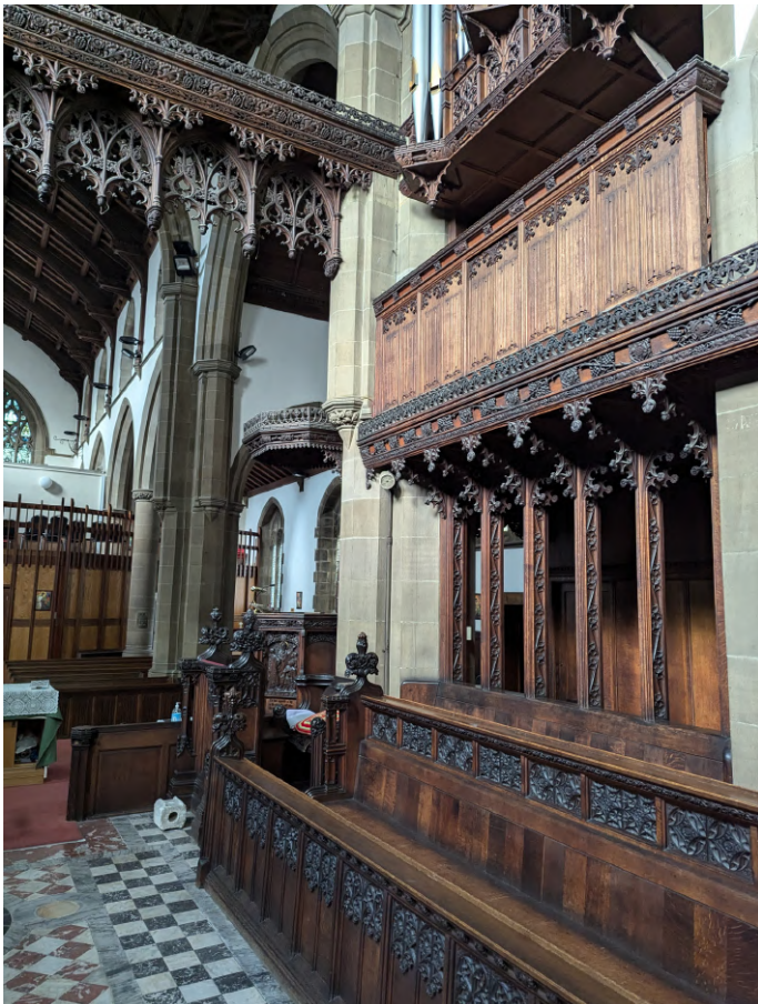
Interior panelling, carved timberwork and metalwork is exceptional and of very high significance.
