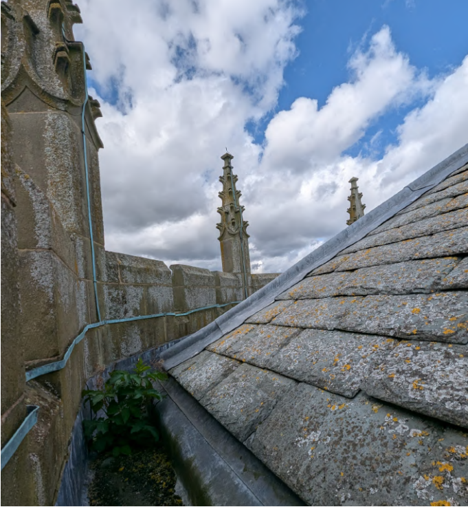
Tower re-roofed in 2015. Good condition. Some build-up of dirt and debris to gutters.
