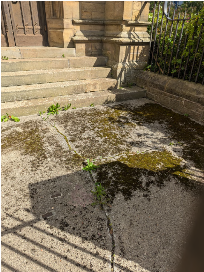
Cracked concrete to front of west door would benefit from repair and steps re-pointed to resist weed growth in gaps. External corners have been lost on some areas of the plinth course around the west door to both sides.
