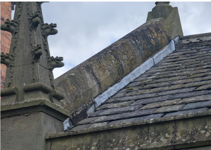
Gable verge of north roof pitch of retro-chapel. Flashings damaged.
