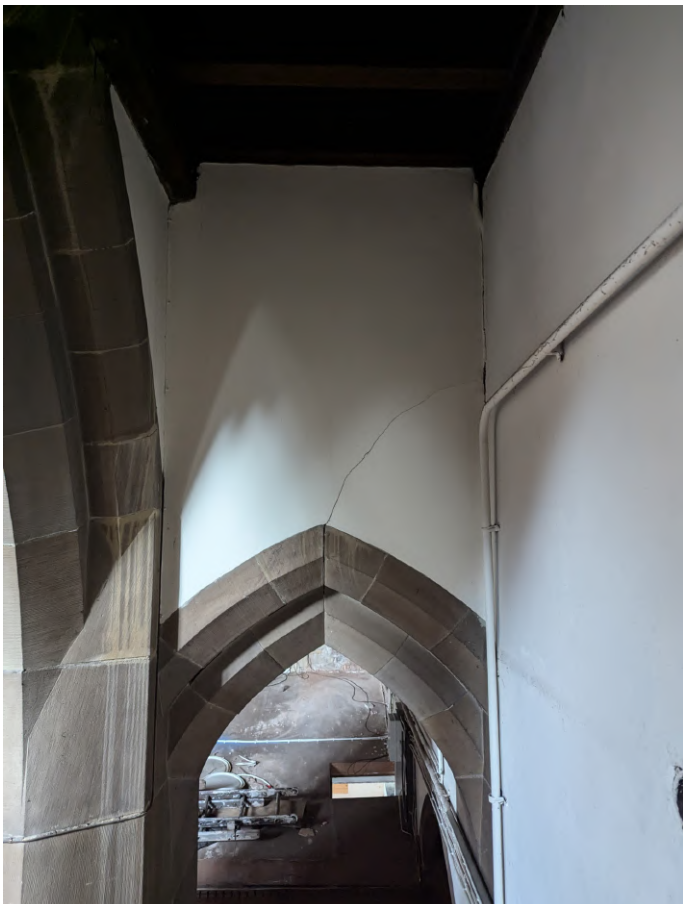
Crack at wall over Angel Loft. East ambulatory.
