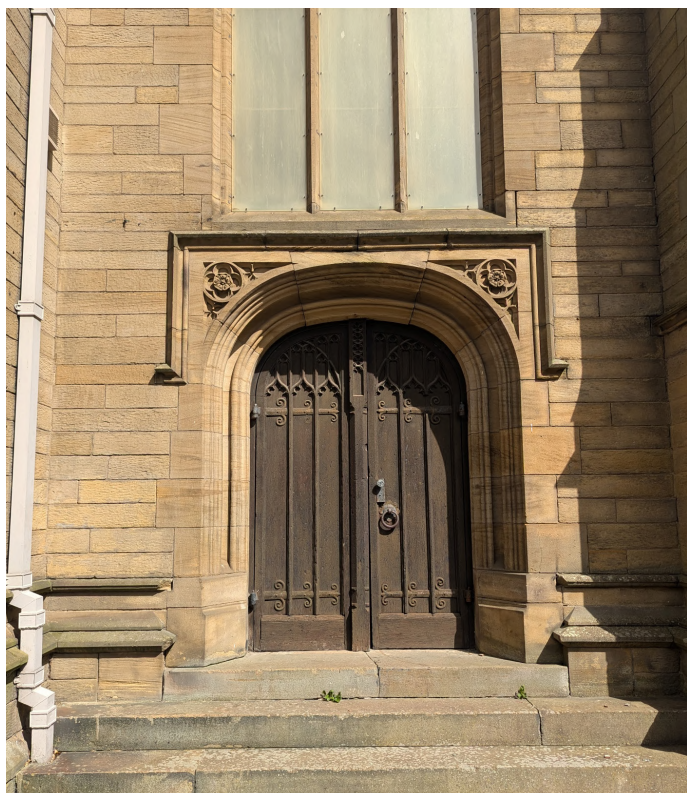
Key stone dropped over main west doorway - not progressed, as per previous QI.
