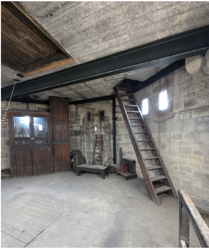
Access to tower roof. Add sign to warn users about the exit onto the parapet so they understand the risks. Clock mechanism behind.
