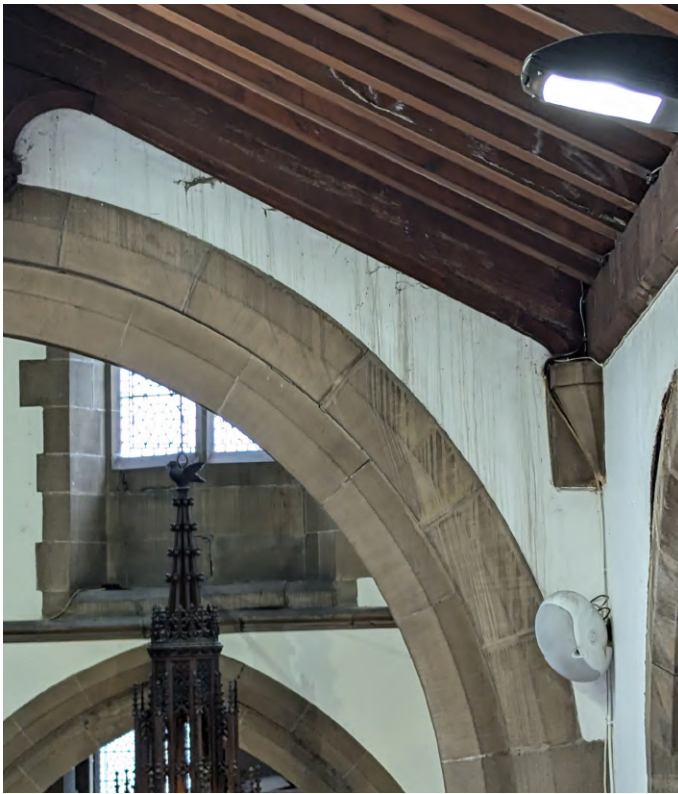
Water staining to wall below south aisle roof abutment with south transept. Now resolved. Monitor area and redecorate.
