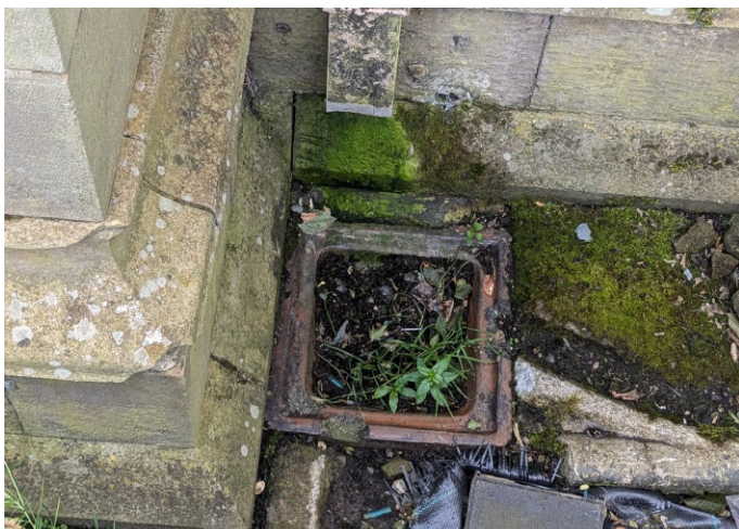
Blocked gully on south side of church. Shoe missing to hopper. Requires refurbishment.
