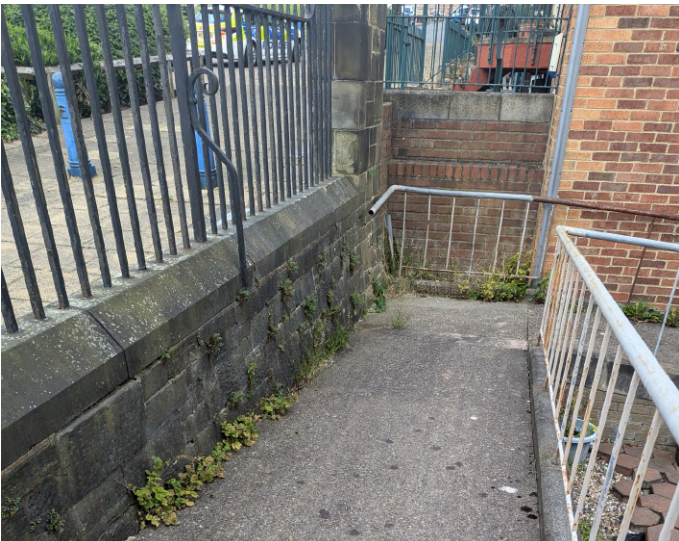
Accessible ramp down to north-east entrance. Railings require some redecoration. Boundary wall requires weeding and repointing.
