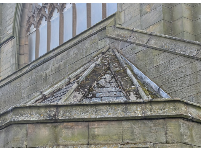
Roof of porch at north-east corner. Parapet over with movement to copings above.
