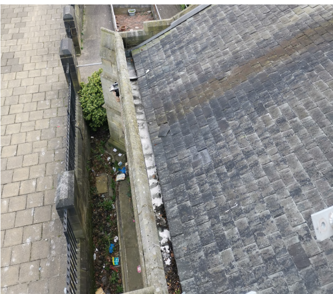
North chancel aisle roof in poor condition, slipped and broken states. Issue with gutters causing water ingress to the choir vestry below.
