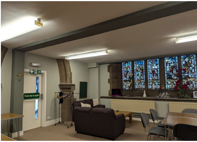
Meeting room on gallery level - ceiling cuts west window in half and creates a low-ceilinged, rather unpleasant space - consider removing the ceiling to allow appreciation of roof and west window (appreciate heating issues will have to be considered).
