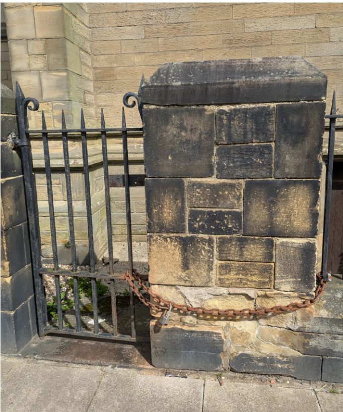
Damage to the stone pier at the west boundary wall due to the large heavy chain securing the west gate. General repointing required and minor indents to damaged stone.
