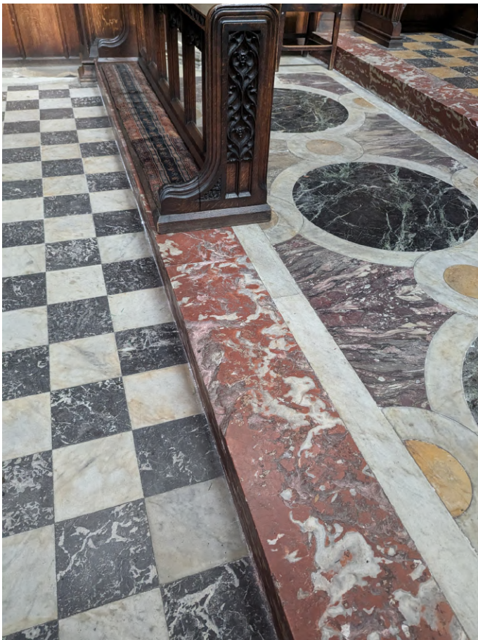
Marble floor to chancel - all interior of exceptional quality. Minor damage to steps.
