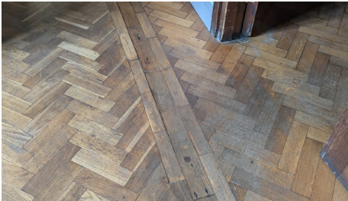
Wear and tear to flooring. Floor would benefit from sanding and re-finishing.
