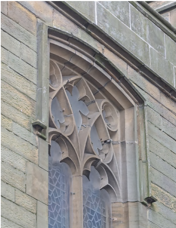
Loss of pointing to fine joints and tracery. Remove mastic and repoint in lime.
