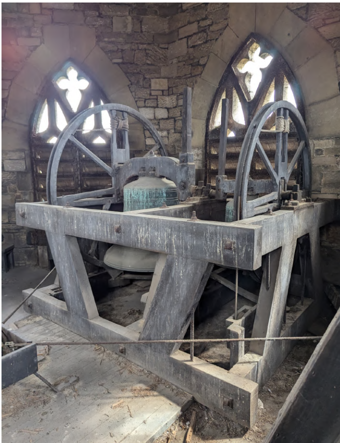
Timber bell frame on concrete floor - good condition though would benefit from a clean
