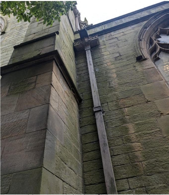
Hopper and downpipe to north aisle roof in better condition than before due to maintenance. Some refurbishment still needed.
