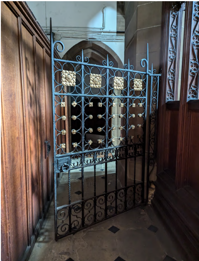
Gate to north ambulatory. Requires some redecoration and refurbishment.
