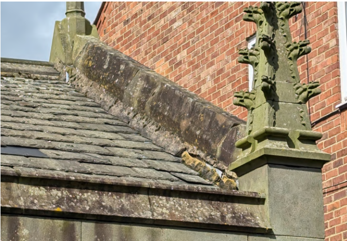
South roof pitch over retro-chapel. Cracking of mortar at verges.
