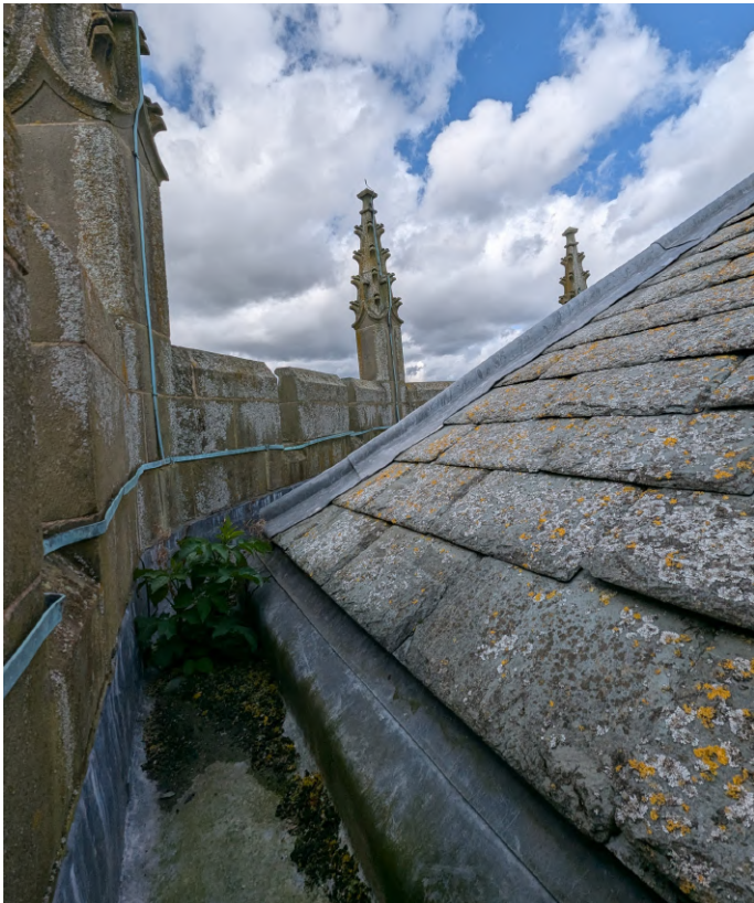
North pinnacle missing lightning rod (upper section)
