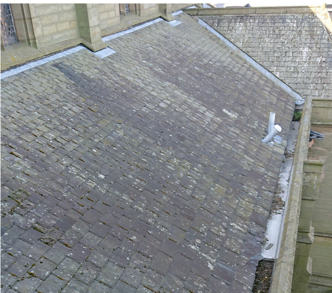
North aisle roof in poor condition. No cowl to vent pipe.
