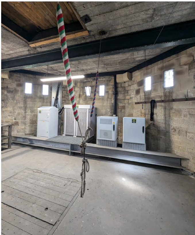
Cellnex telecom installation to first floor of tower.
