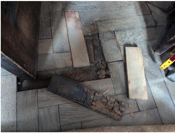
Rot to woodblock flooring at entrance to choir vestry.
