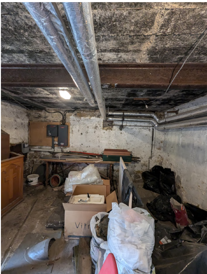
Boiler House - rusting to support beams.
