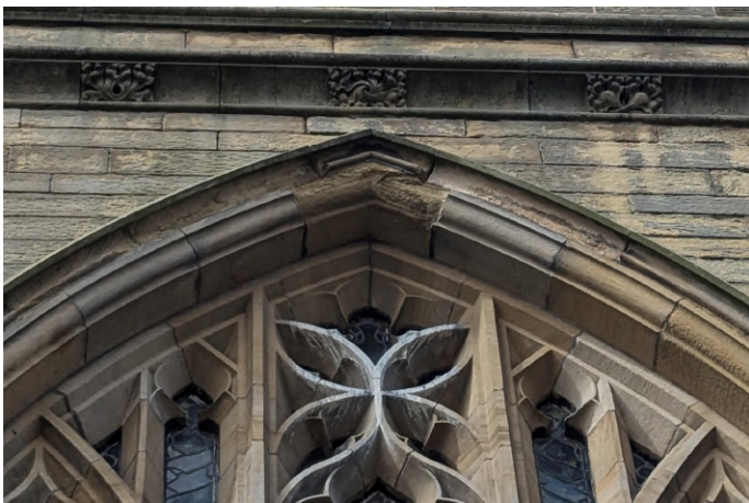
Decay to hood moulds of east window. Guano staining. Loss of pointing to fine joints and tracery.
